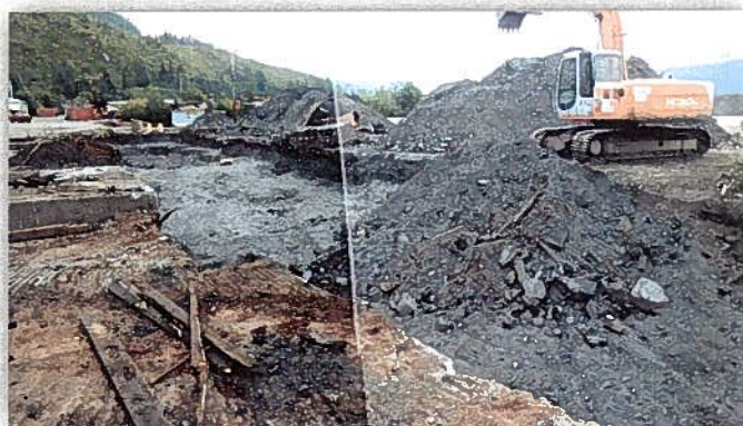
Figure 9: View on 8/21/12 looking toward the south-end of the former cherry picker line.
