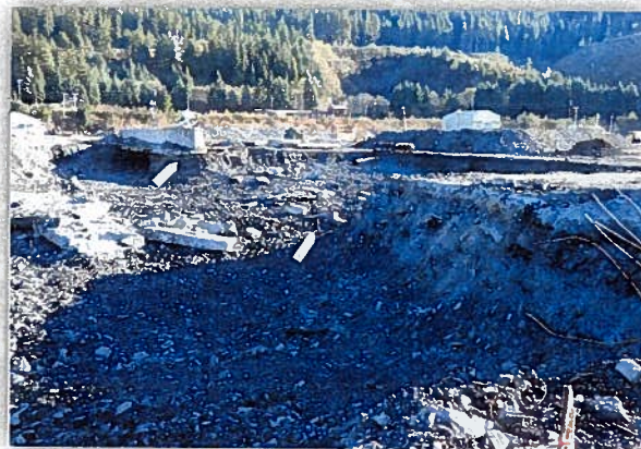
Figure 13: The 10/24/12 view of the log barker area. Arrow in the back shows the log kickout structure and lower arrow indicates the point of origin.
