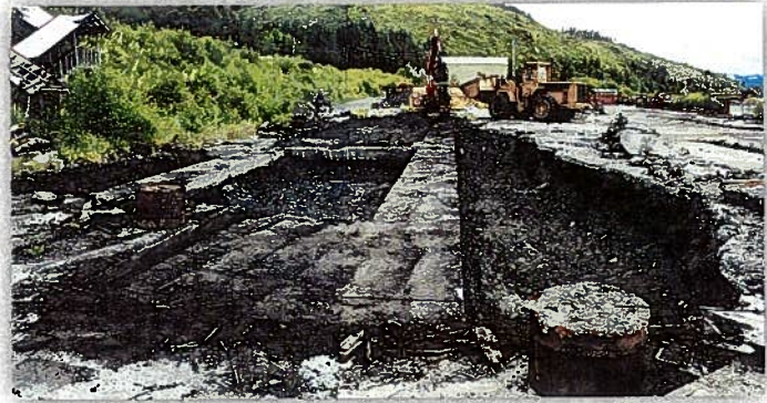
Figure 6: Looking south along the former green chain line area on 6/29/12. Excavations exposed 4'-wide foundations which later were discovered to be the former hydraulic-powered 'action pack'
