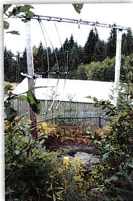
Figure 11: City-Tie Transformer Pad
