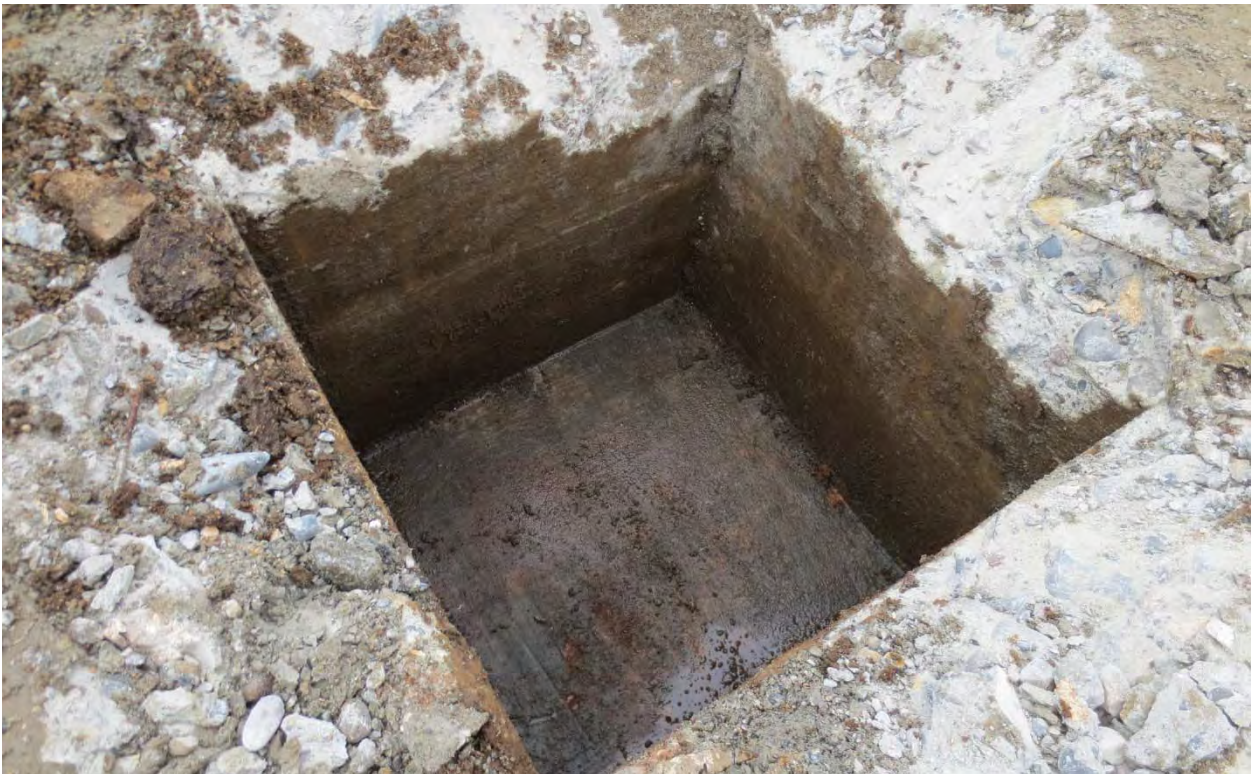
Photo 10: One of two sumps that formerly discharged to a decommissioned septic crib (September 2, 2014).
