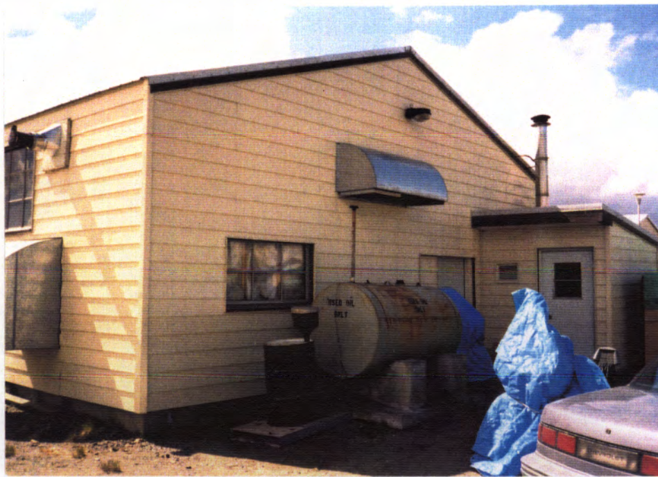
ABOVEGROUND STORAGE TANK (AST) 19-D-5 AT THE SHOP BUILDING 300, VIEWING SOUTHWEST.
