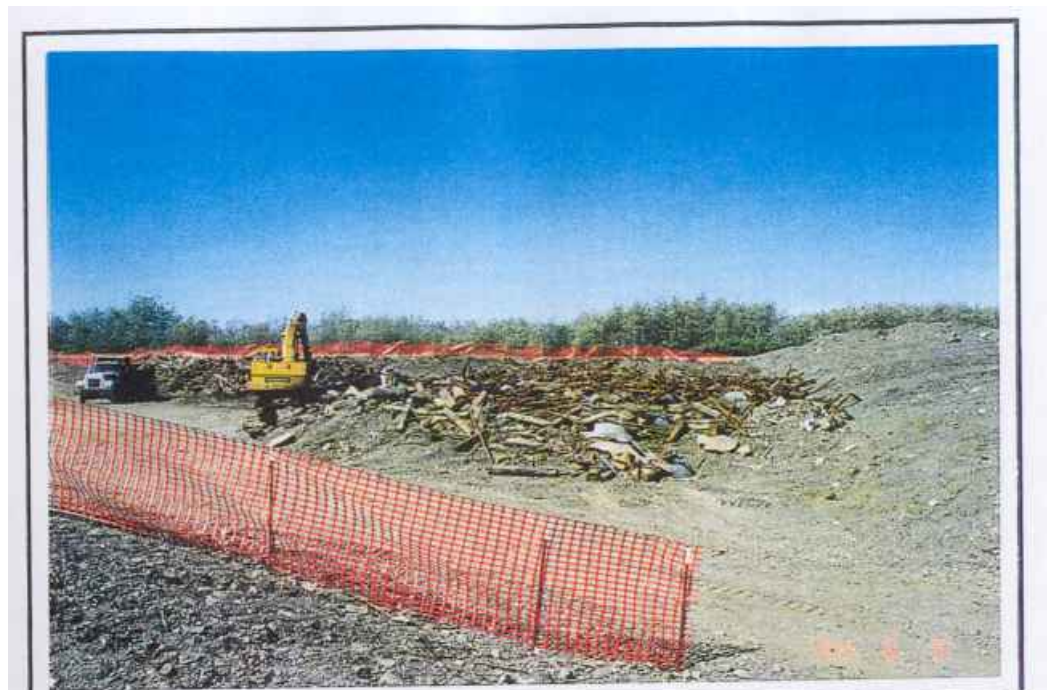
Prison Site "A" Nome Area Sites Project 1994 Work Season - June 9, 1994 Contract DACW41-89-D0133 Eastern Area, landfill operations, view looking west
