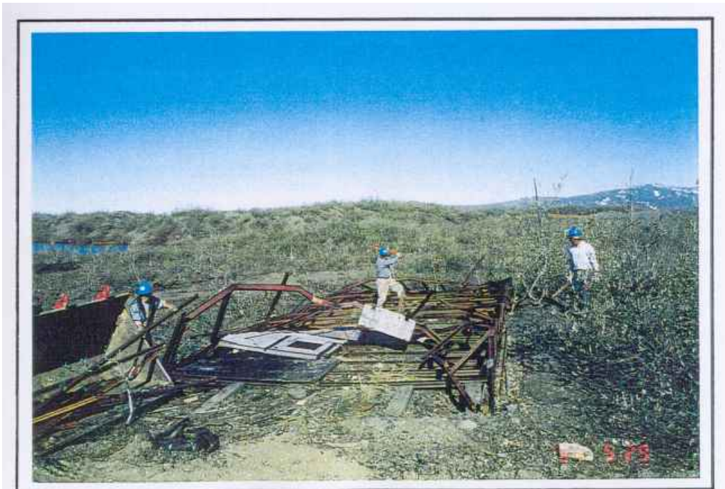
Prison Site "A" Nome Area Sites Project 1994 Work Season - May 29, 1994 Contract DACW41-89-D0133 Eastern Area, Quonset hut demolition
