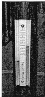
Photograph 3: The U-shaped manometer with the right side red oil shown above zero (proper working condition).
