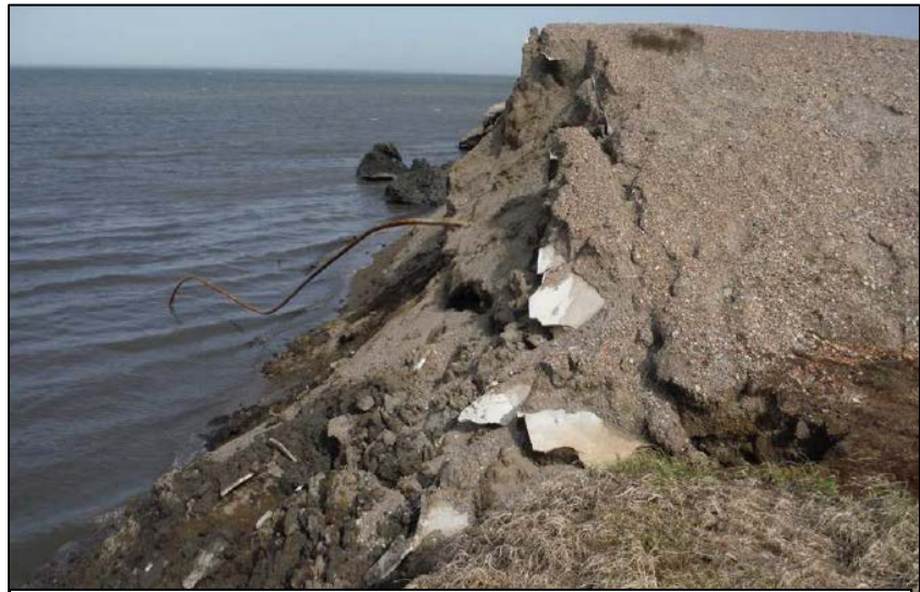
Pipe protruding from berm at beach showing Styrofoam beneath surface of berm (2014 photo courtesy of BEM).
