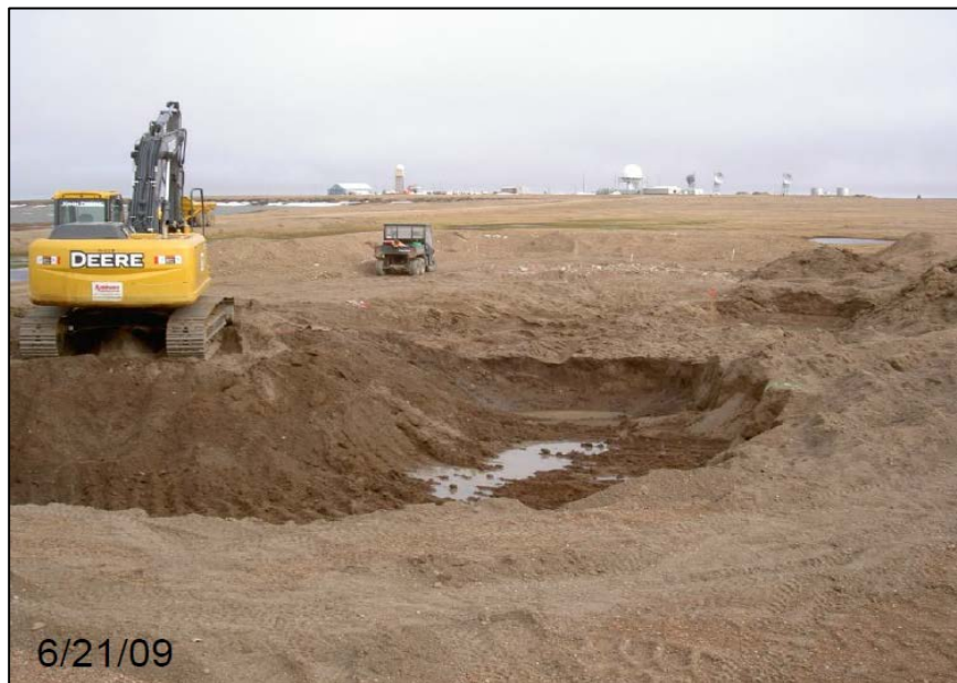
Initial excavation of Beach Diesel Tank northern area was advanced to the frost line at approximately 2.5 feet below grade (2009 photo courtesy of BEM).
