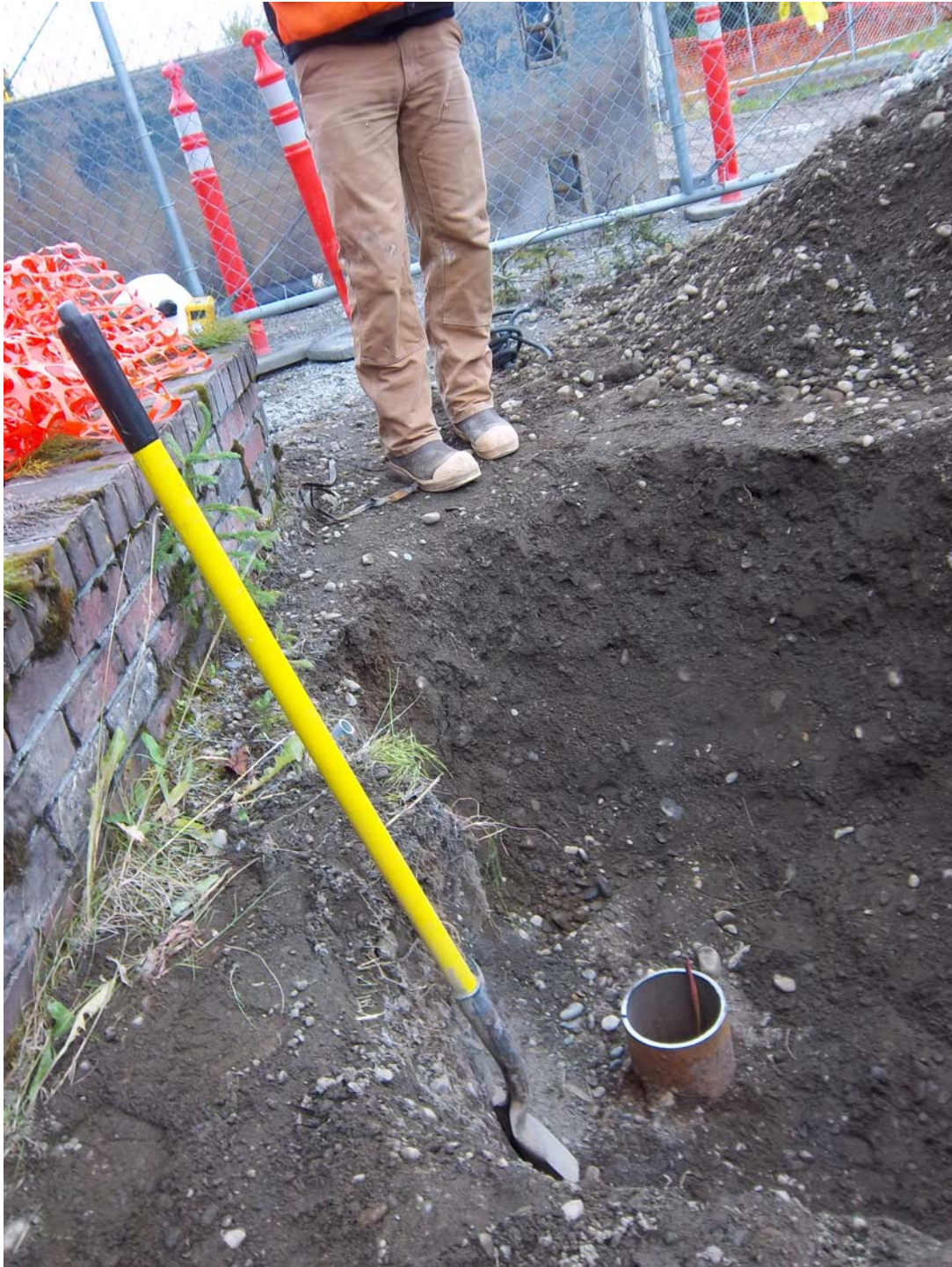
PHOTO 2 – Potable water well casing cut approximately 2 ft bgs.
