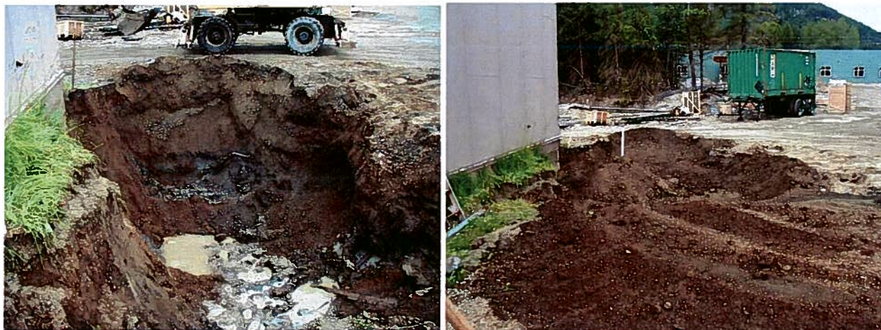
Stained grey soil layer in the north wall and groundwater monitor well emerging from clean backfill soil.
