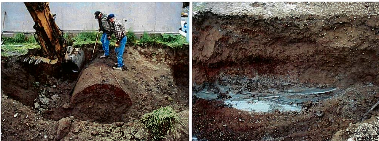
UST at the northeast corner of the Vo-Tech building; subsurface clay layer and groundwater seep.
