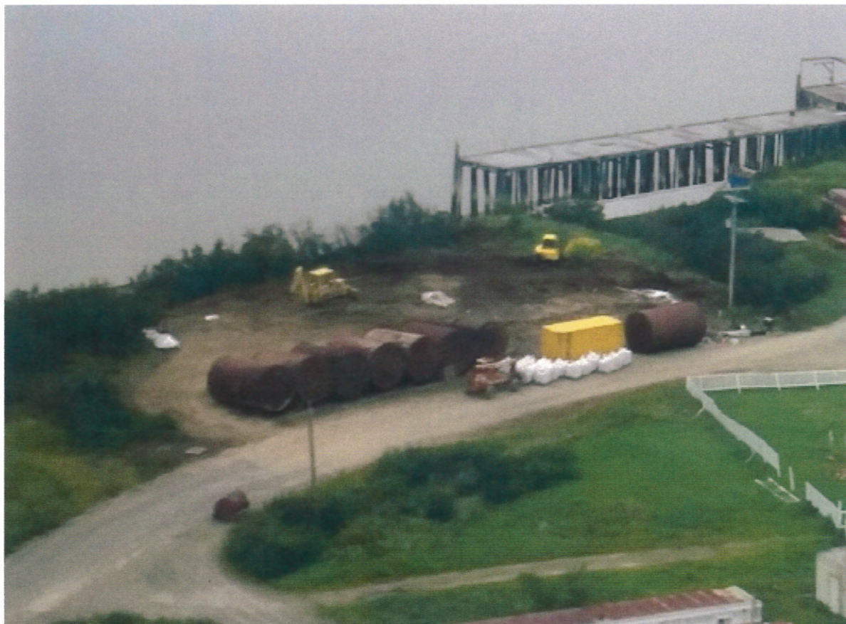
Figure 1.2- 2013 aerial photograph looking northeast of site after excavation, Super Sack filing, stockpile construction, and tank arrangement (G-logics 2014 Cleanup Action Report).
