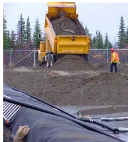
Pipes buried in the soil increase air circulation and speed the action of bacteria which break down the contamination through biological processes. (DEC photo)
