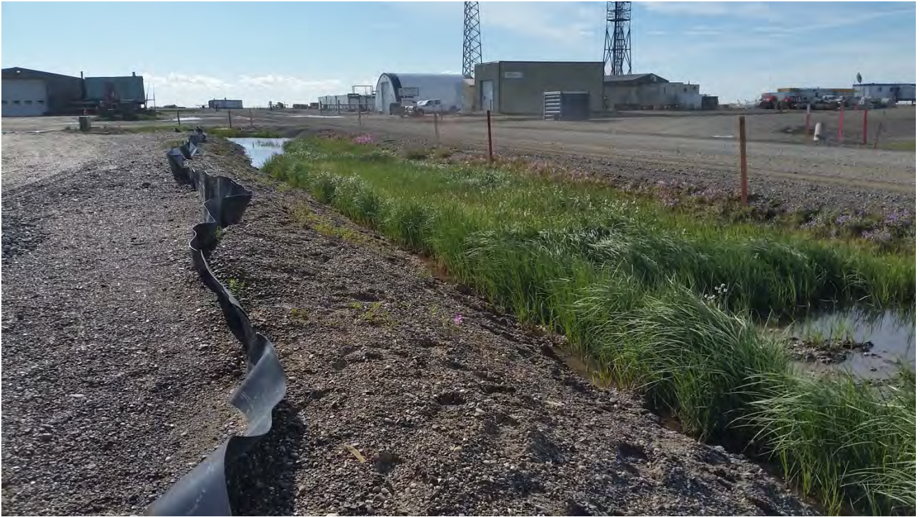
Photo 1: Intact pad liner along the northwest edge of the north pond. Photograph faces northwest.
