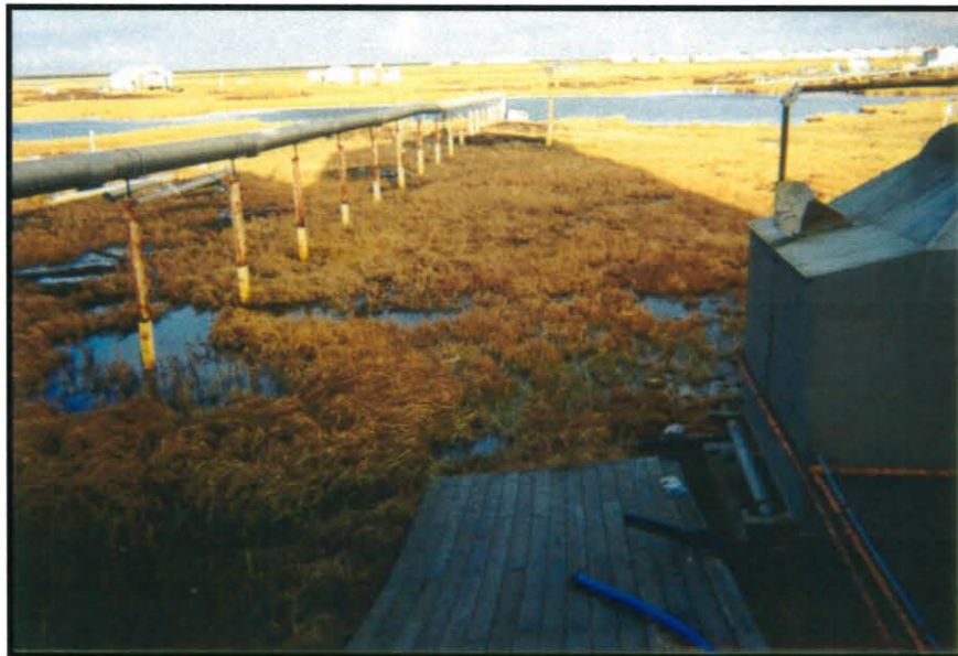
Village: Kwigillingok ADEC Site Number: 2 Site Name: Kwig Incorporated, Washeteria Direction: E Description: North end of the AST. The Washeteria lagoon is in the background.
