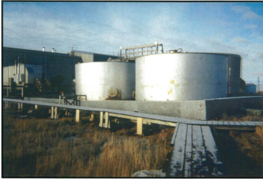
Village: Kwigillingok ADEC Site Number: 1 Site Name: Kwigillingok School, LKSD Direction: NW Description: Two ASTs at the school's tank farm.
