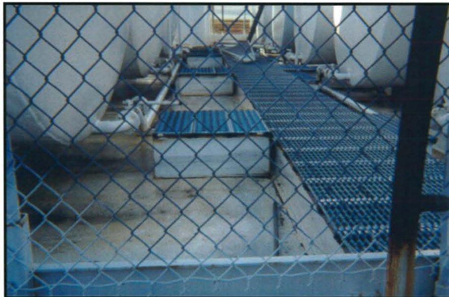
Village: Kwigillingok Photo 10 ADEC Site Number: 4 Site Name: Kwig Incorporated & Kwigillingok Village Council, Powerhouse and Retail Sales Direction: E Description: The floor of the tank farm. No spills or leaks are visible.
