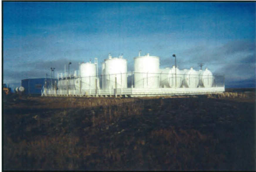
Village: Kwigillingok Photo 9 ADEC Site Number: 4 Site Name: Kwig Incorporated & Kwigillingok Village Council, Powerhouse and Retail Sales Direction: SE Description: Tank farm. The Kwigillingok River is located approximately 400 feet east of the tank farm.
