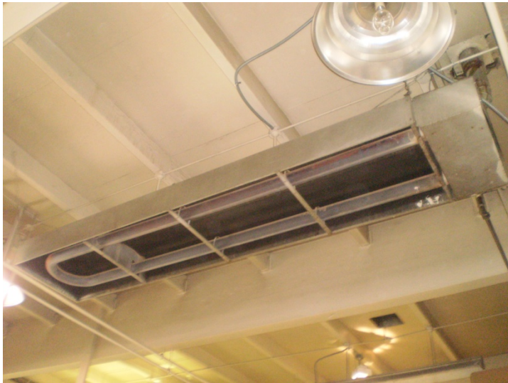
Photo 3. Heater Located in Western Portion of Garage
