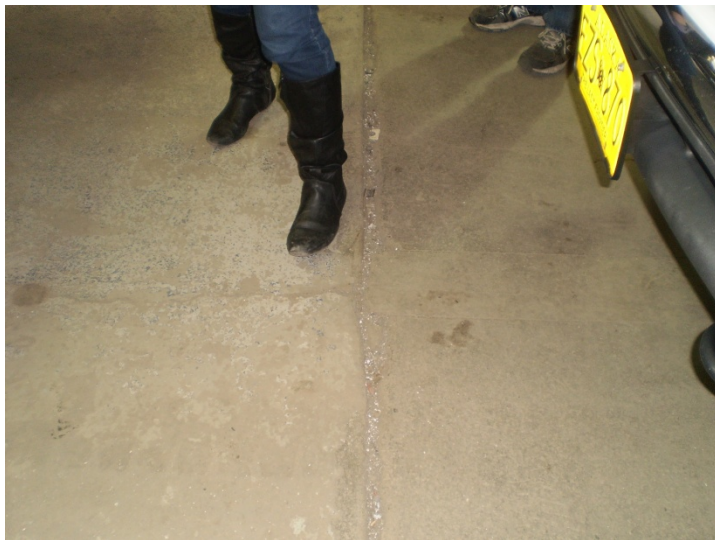
Photo 5. Crack in Concrete Between Garage Areas
