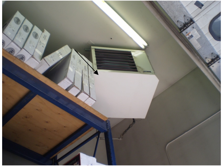
Photo 2. Heater Located in Eastern Portion of Garage
