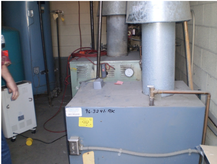
Photo 9. Boiler Room Near Northwestern Portion of Building. The boiler is no longer in use.
