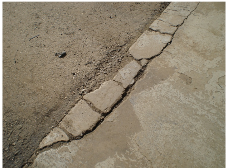
Photo 6. Crack in Concrete Between Garage and Outside Wall
