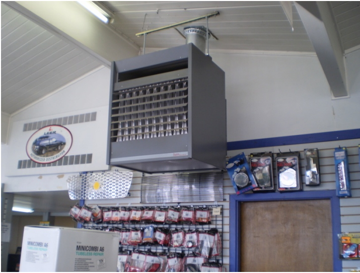
Photo 1. Heater Located in Showroom
