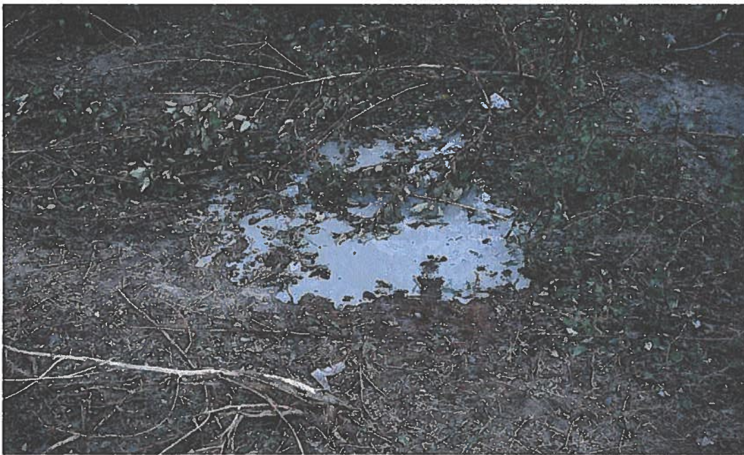
48. SVE-4 Location of horizontal well where grout daylighted by pressure.
