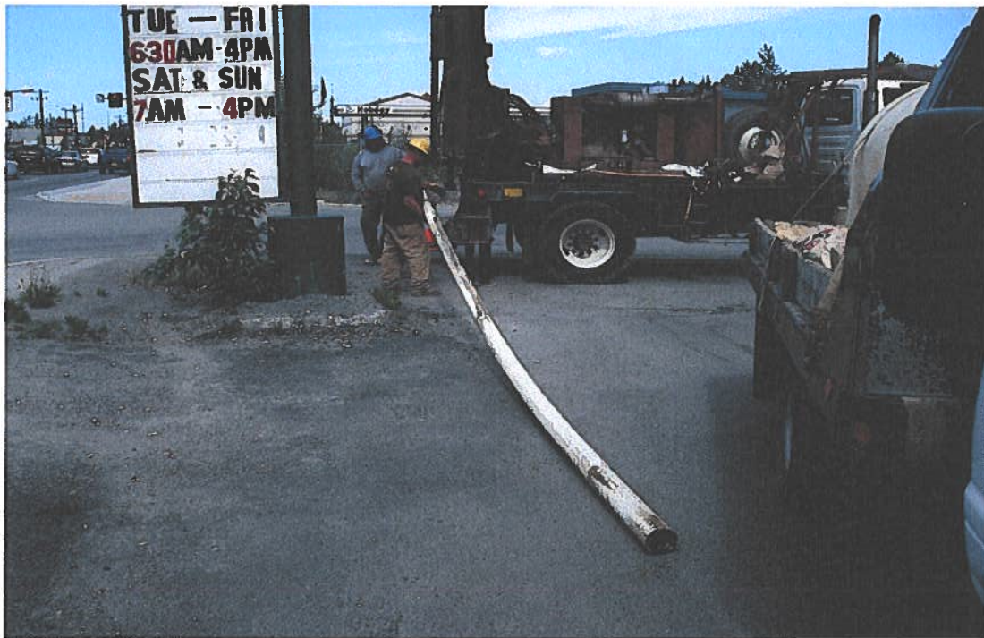
14. MW-6 Showing the well casing bottom cap knocked out.
