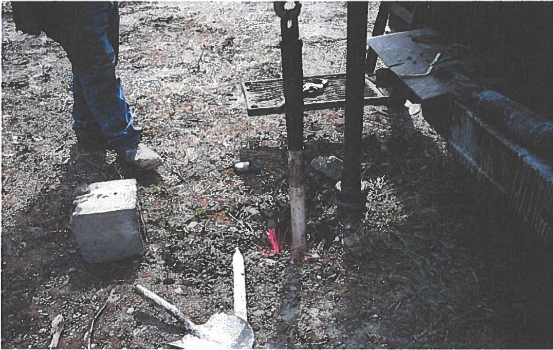
47. SVE-3 Pulling well casing with a taper tap, protective vault to left.
