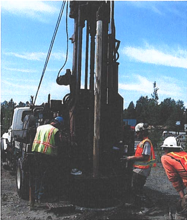
37. CW-2 Casing broke off at screen, 12 feet below ground surface.
