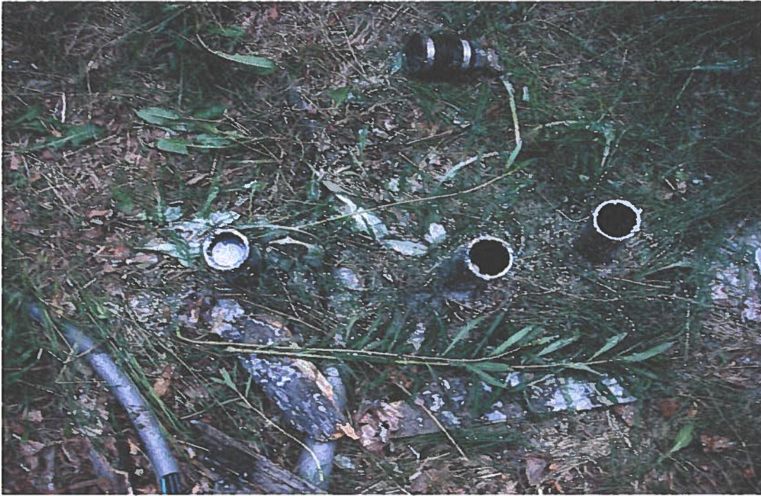
43. SVE lines stabilized; these lines were later cut off flush with the ground surface.
