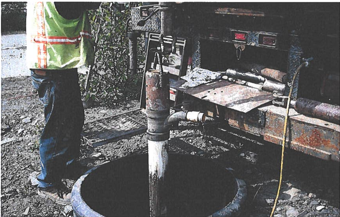
34. CW-1 Pulling the well casing with a fabricated metal sleeve and self tapping screws .
