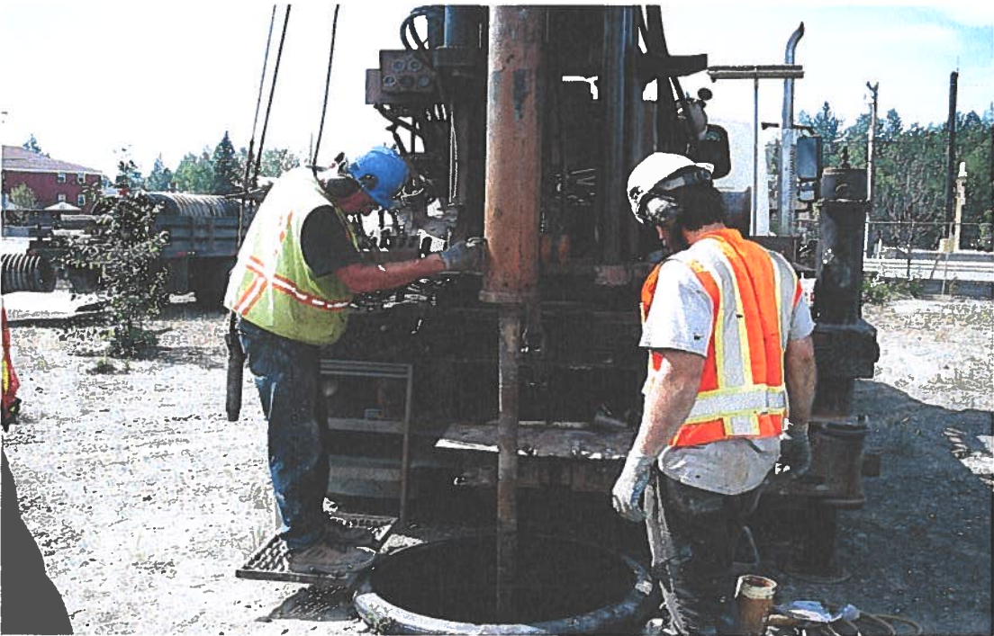
36. CW-2 Knocking the bottom out of well casing with a drill rod.
