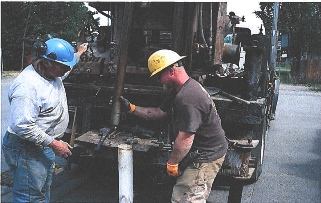
10. MW-5 Using the drill rig's center rod to knock out the bottom of the well casing.
