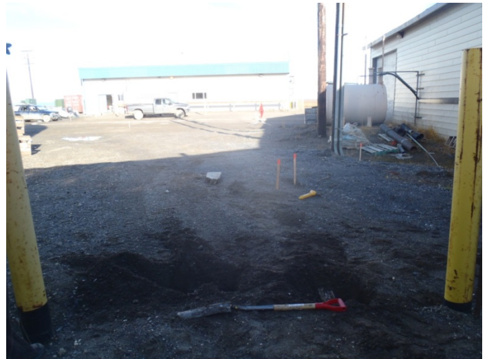
6) Area of contamination, facing west.
