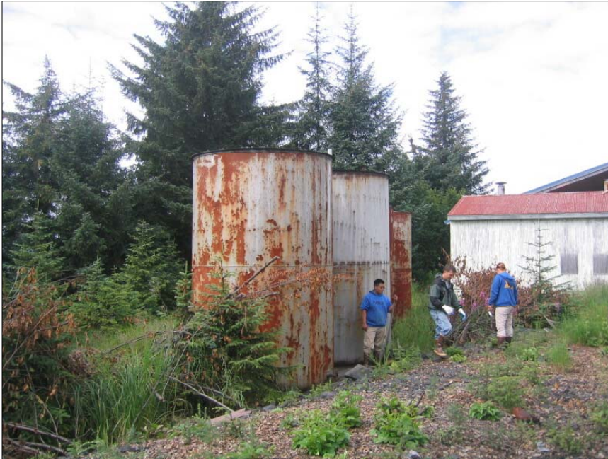
PHOTO 1 Old Tanks at Area A looking northwest. Generator complex "shot rock" pad in foreground.
