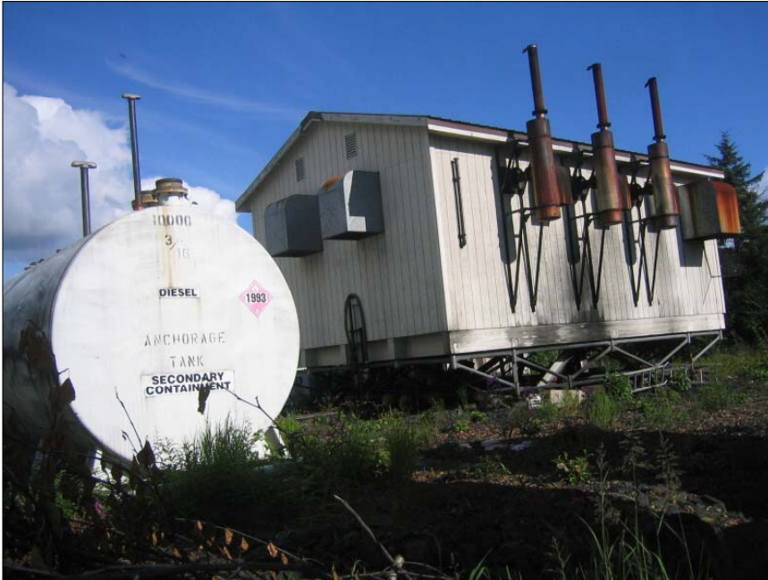
PHOTO 3 New 10,000 Gal AST and generator building looking south east from edge of old tanks.
