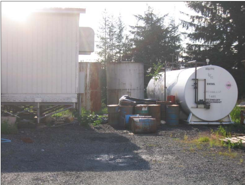
PHOTO 4 New 10,000 Gal AST and generator building in background looking west. Note drums near the AST
