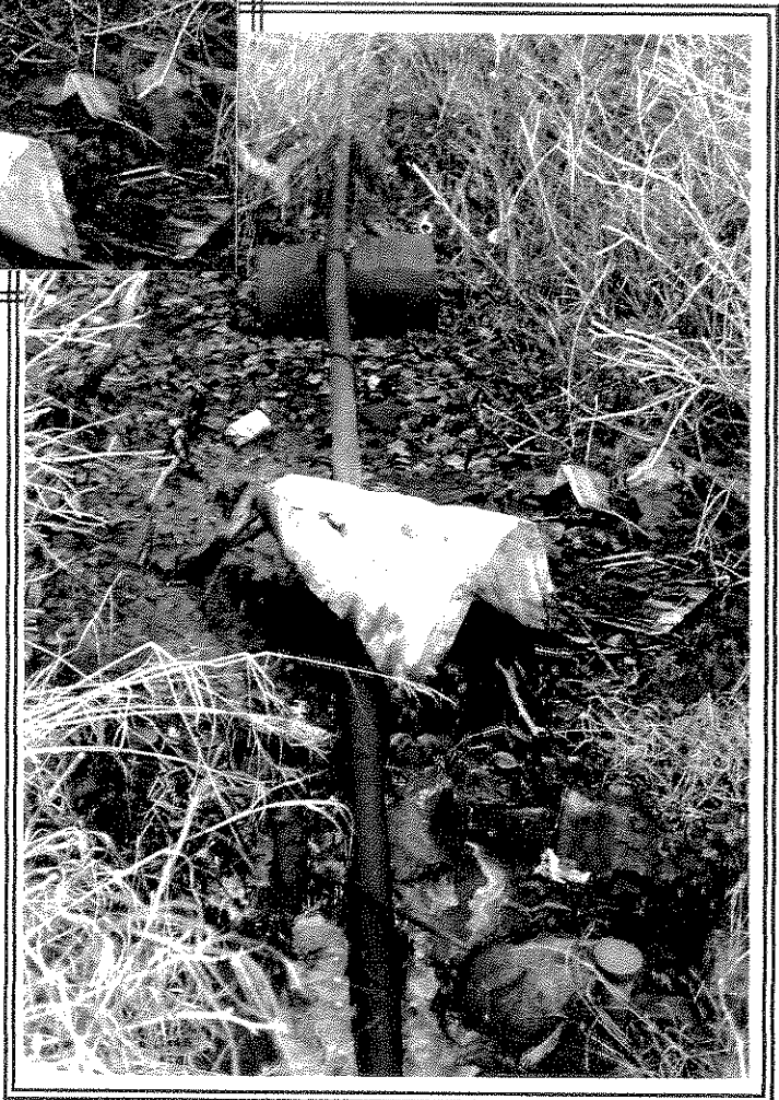
Picture 6: Stained area around 3" dia. fuel line.
