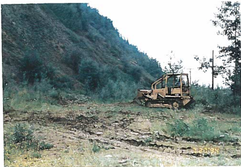
Photo 6: Preparation of impacted soil stockpile area included the removal of debris and site grading.
