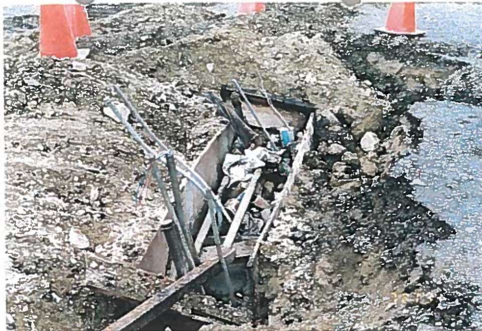
Photo 5: Close-up view of dispenser area underground piping.
