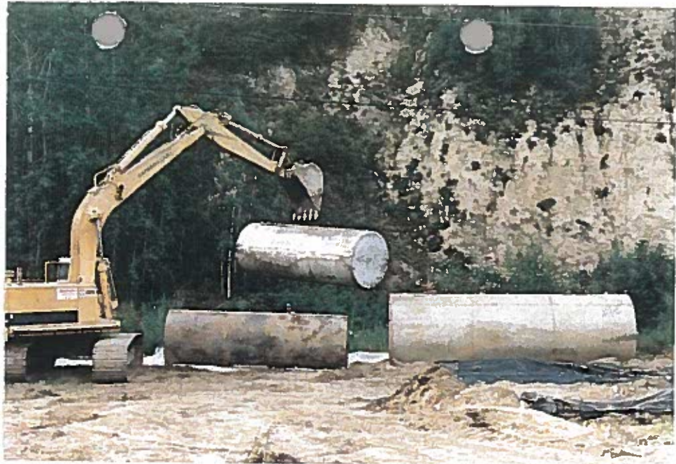
Photo 25: The tanks were stored on 10-mil polyethylene liner adjacent to the impacted soil stockpile.
