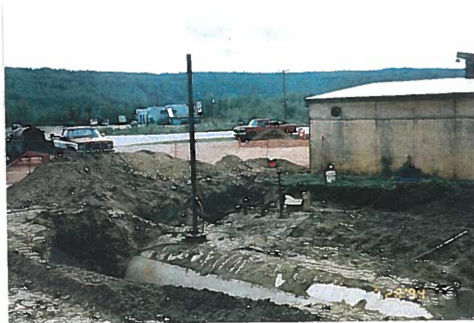
Photo 16: The tanks were purged with air and were subsequently inerted with dry ice.
