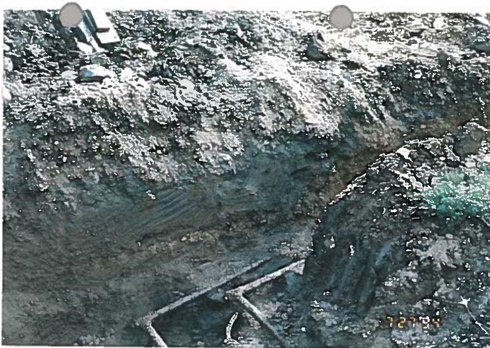
Photo 9: Grey-stained soils were observed to extend to approximately 8 feet below grade, dissipating laterally away from the fill piping area.
