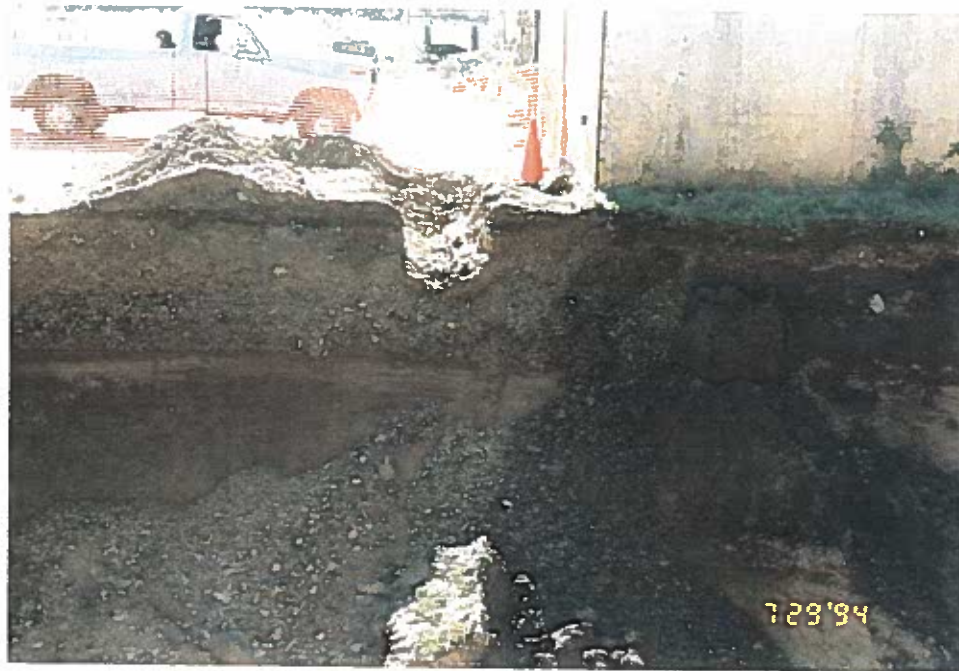
Photo 27: Soil conditions along the western sidewall of the tank area, adjacent to the store building.
