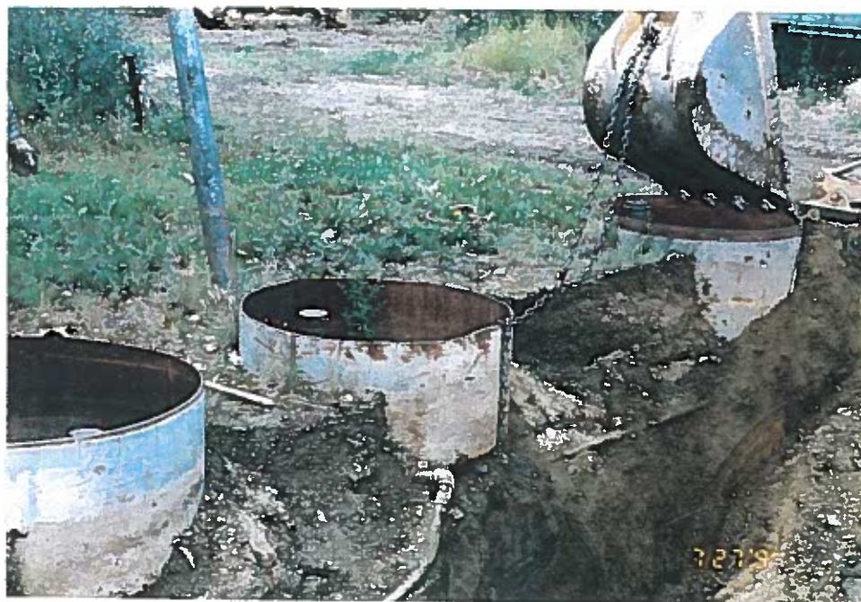
Photo 10: Protective metal casings were removed from around fill pipes during site work.
