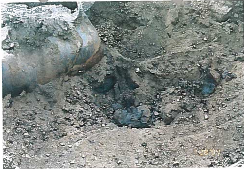
Photo 21: Grey-stained soils were observed on the vent end of Tank No. 2.
