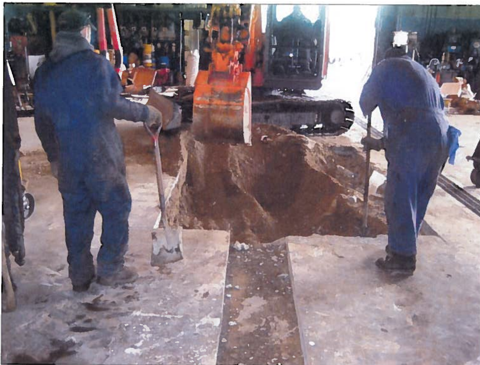
Photo 02 - Start of excavation for dry well structure removal and oil water separator system installation
