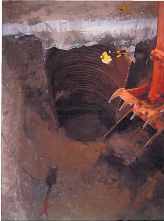
Photo 05 - Removal of remaining sludge from dry well structure, remainder of dry well structure left in place to support concrete floor and trench drain
