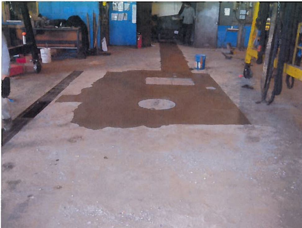
Photo 10 - Completion of oil water separator system installation with monitoring well located in the small monument on the right
