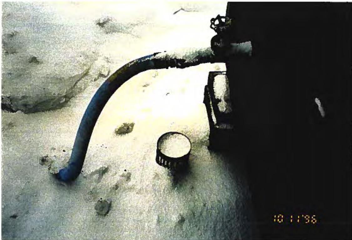
Rear of Jet A Fuel Cabinet (Looking West) 10-11-96
