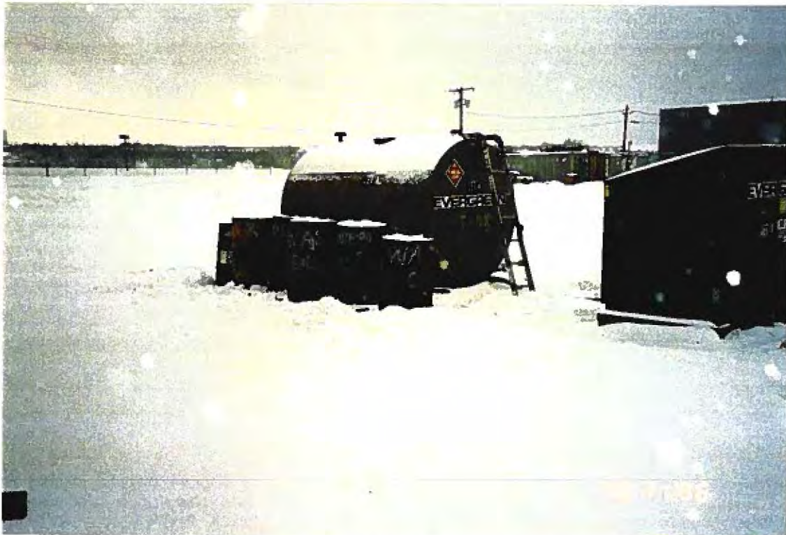
2000-gallon AST and Fuel Dispenser Cabinet (Looking South), 10-11-96
