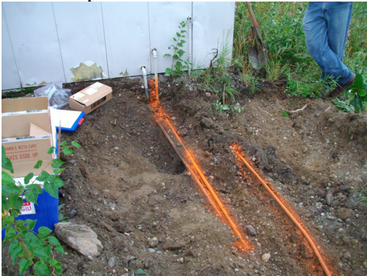
Photo 9. Fuel Delivery Line and Electrical Conduit
