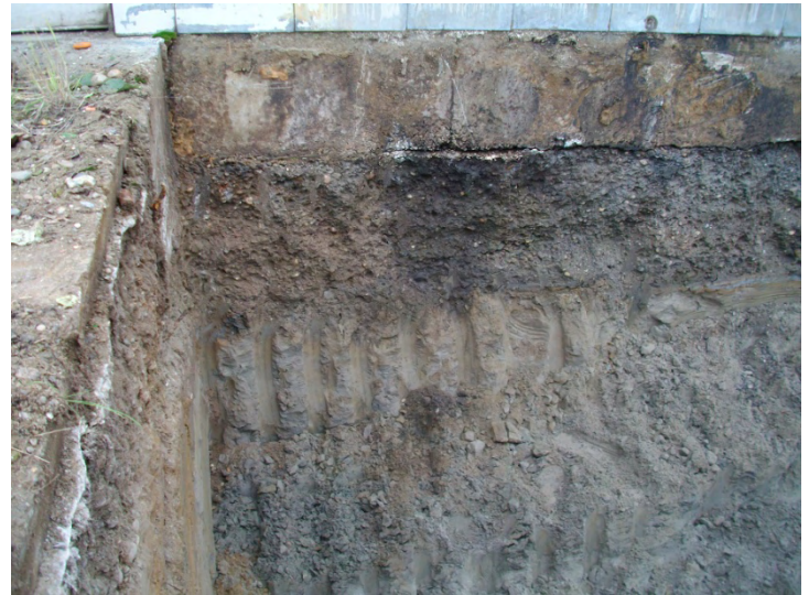
Photo 4. Contaminated Soils Beneath 4-Bay Building
