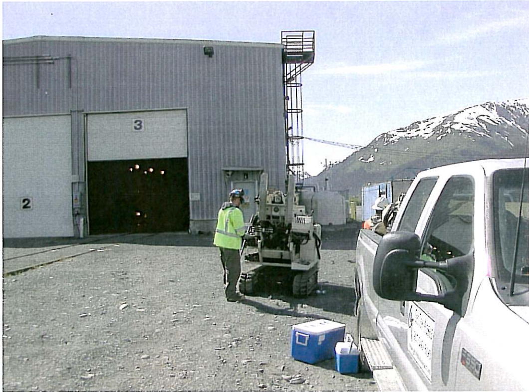
Photograph 1: Installing temporary monitoring well MW-1 50 feet north of Roundhouse, view looking south.
