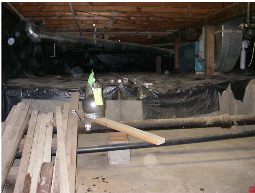
Photograph 2. February crawl space air sample CS-1.
