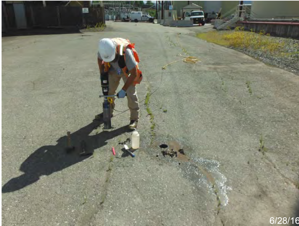
Photo 11. Collection of soil samples underneath pavement in the current asphalt area planned for removal. A 3-inch coring drill was used to remove pavement and reach the soil underneath. Sample location AP-AA15 is shown. Photo faces east.
