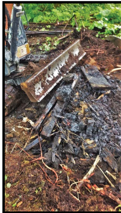
Photo 4: Some buried lumber was discovered among the contaminated soil. It also was coated heavily in the petroleum waste.
