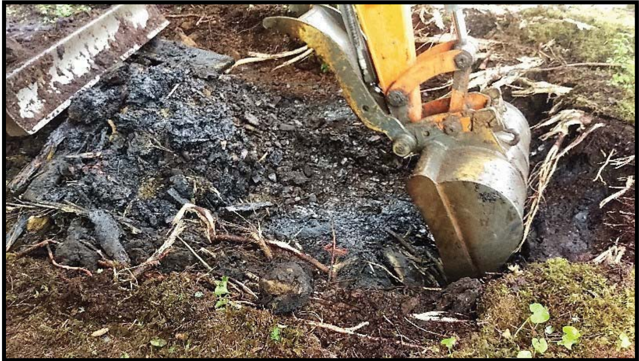
Photo 5: Excavation on north end of site. Note black staining of soils and shot rock.
