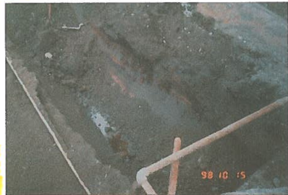
Pooled product in bottom of heating oil UST excavation.
