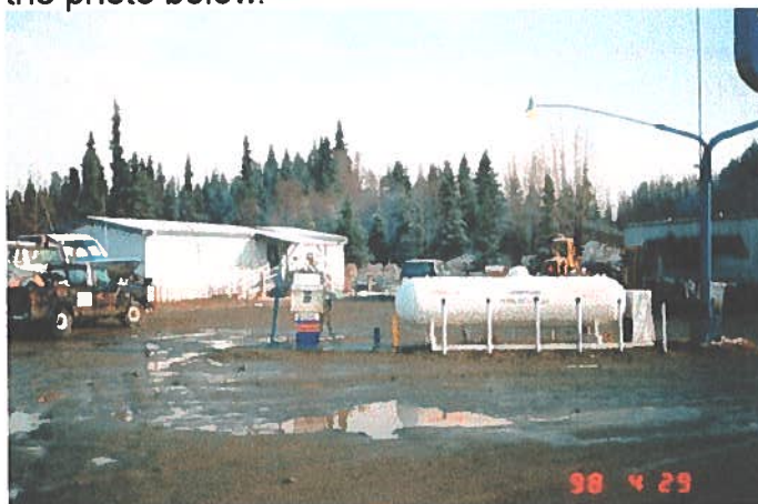
Diesel dispenser island.
