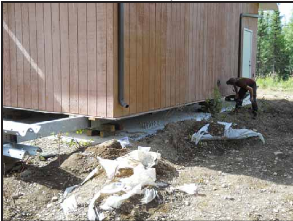
Photo 3: During building removal in vicinity of former location of heating fuel AST.
