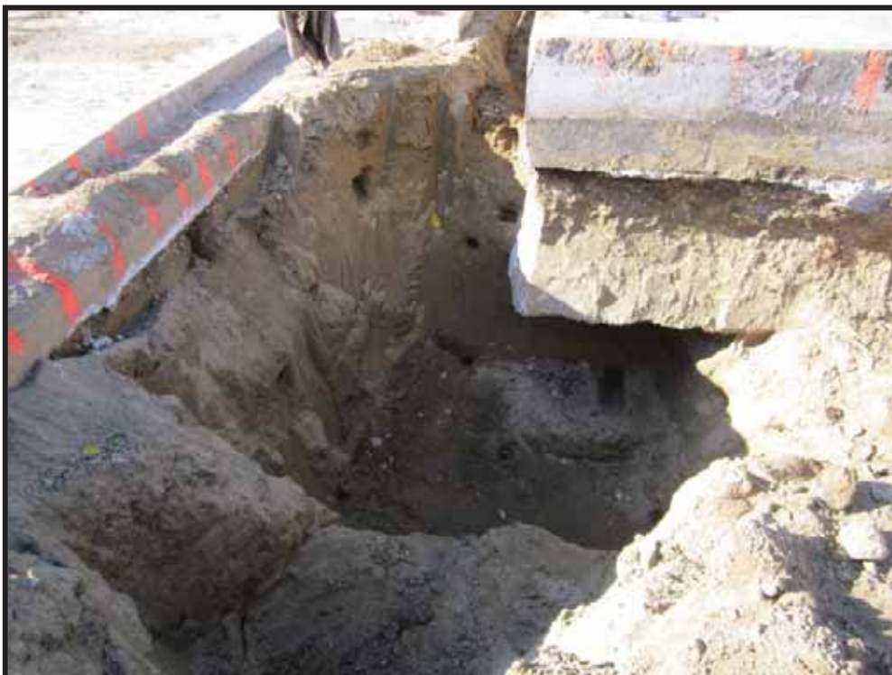
Photo 6: Final limits of excavation between footing perimeter and generator pedestal. Orange markings are 1-foot demarcation lines.
