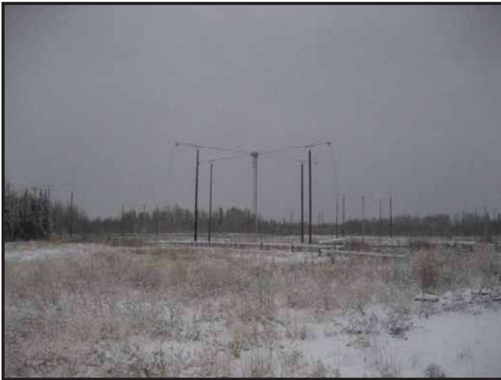
Photo 1: Looking east at original Main Transmitter Antenna Array. All piping, antenna, anchors, and ground grid materials have been removed (2008)
