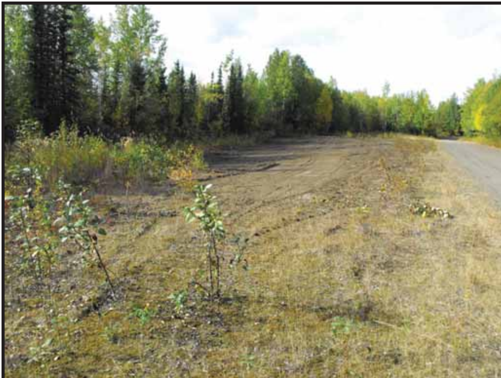
Photo 8: Looking west at loading dock area after removal of all materials and debris (2012)
