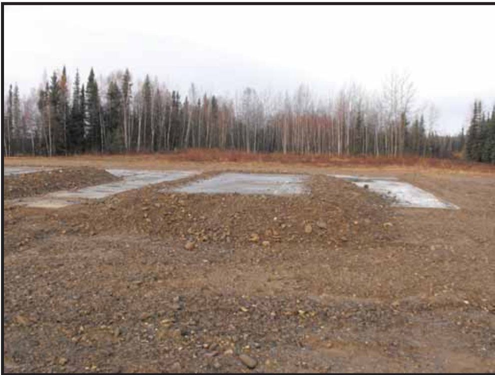
Photo 2: Final grading of site with Generator Building foundation in foreground and former septic tank location in upper left.
