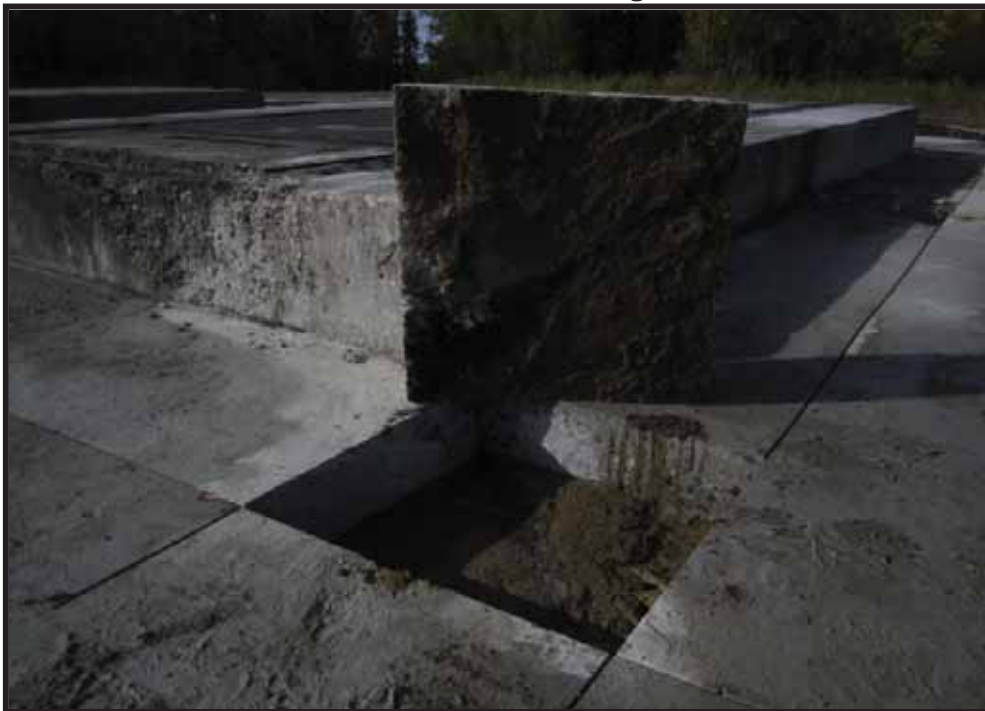
Photo 3: The concrete around the central and north generator pads in the former powerhouse was cut in a two foot wide perimeter around the pads. Typical cut around generator pedestal for assessment.
