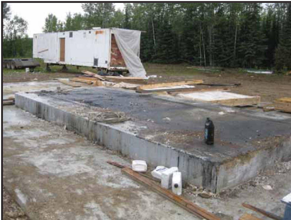
Photo 2: North generator pedestal after removal of generator and Generator Building. Stained concrete from release of fluids during removal.
