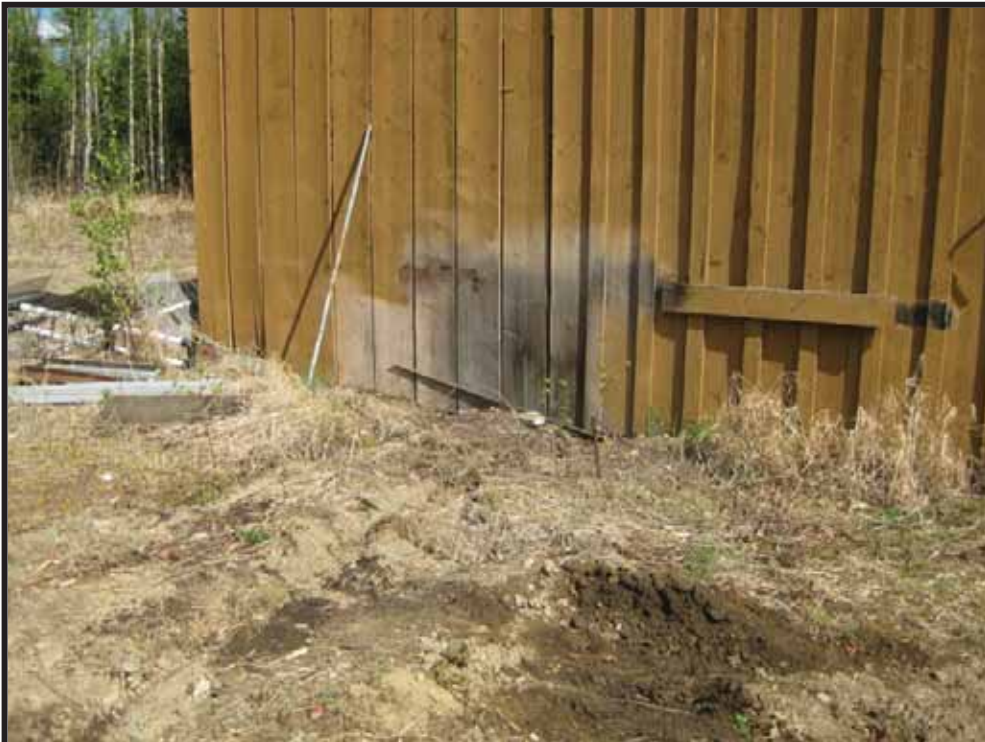
Photo 2: Photo taken facing south showing staining in the vicinity of the former location of the heating oil AST and to the north.
