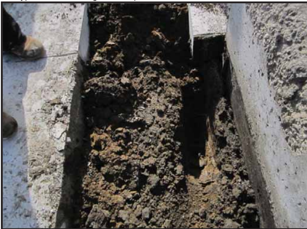
Photo 4: Hydrocarbon odor and evidence of staining on southeast corner of north generator pedestal during initial assessment. Additional concrete removal necessary.
