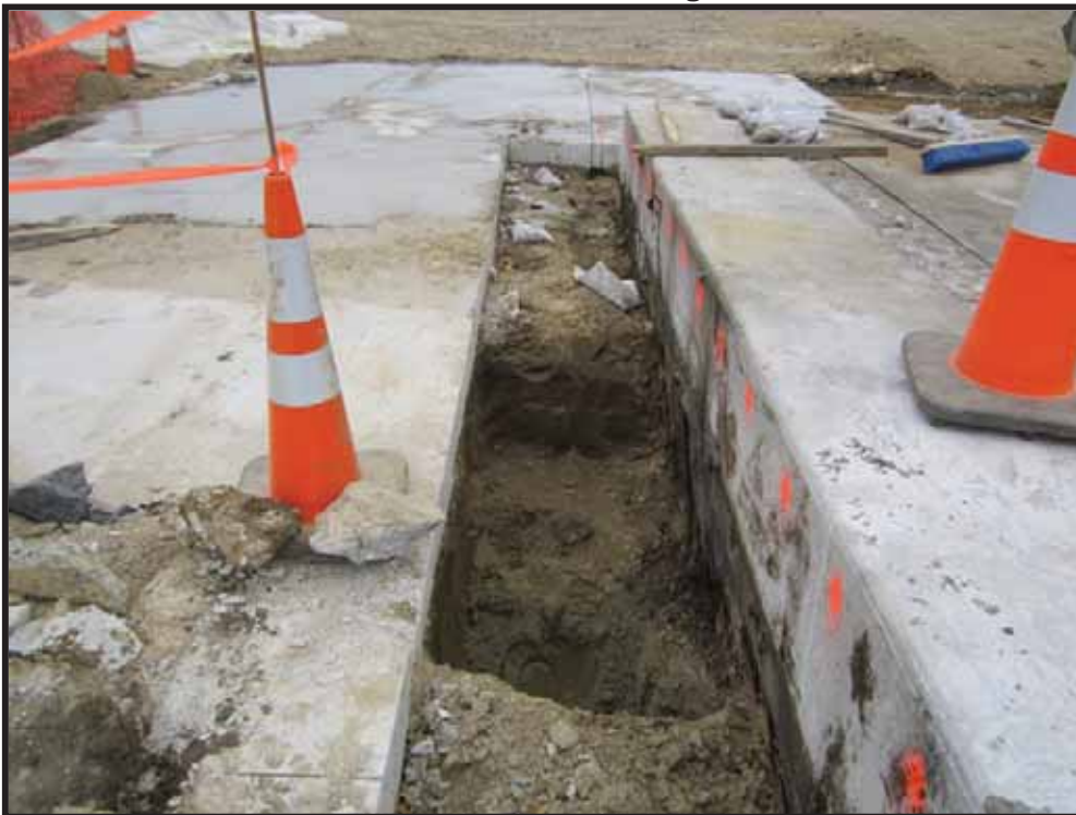
Photo 9: Hand excavation of stained soil on north side of central pedestal, typical of perimeter lubrication oil stains.
