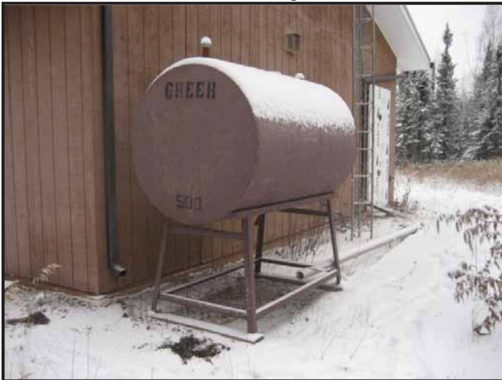
Photo 1: Above ground fuel tank at north end of LIDAR building that was reputedly overfilled (2008).
