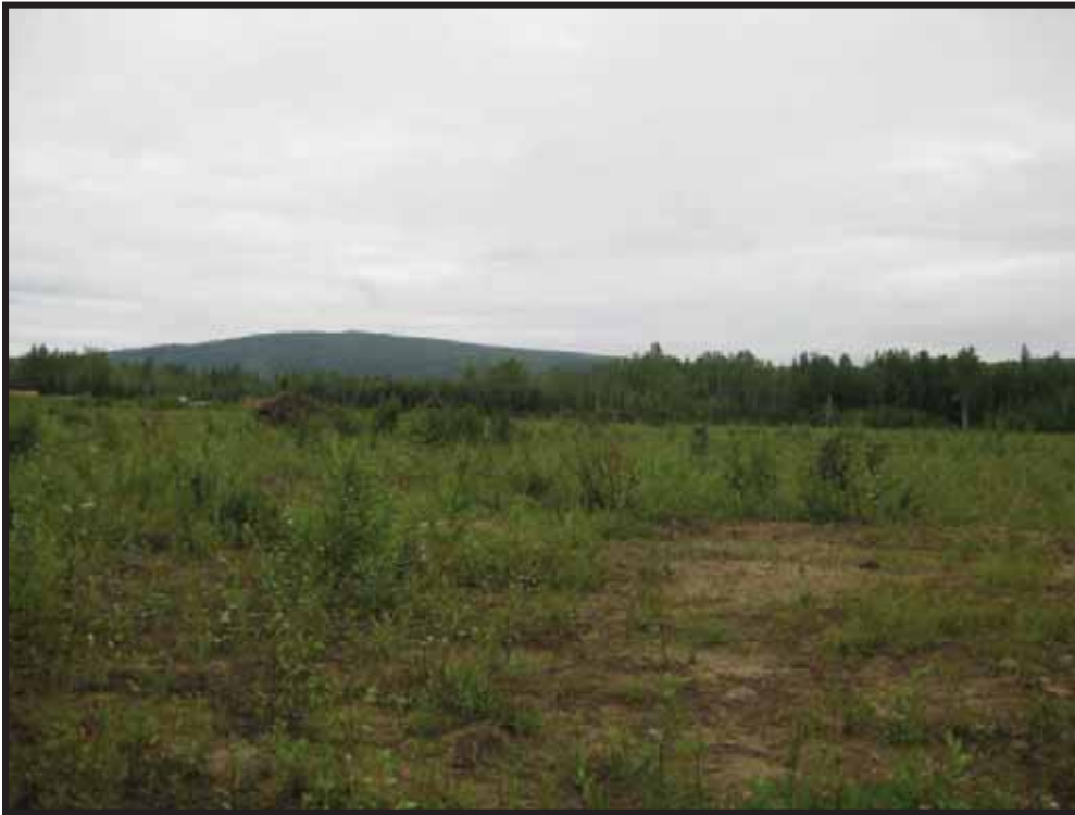
Photo 3: Looking southeast across Main Transmitter Array Area after removal of antenna with bundles of grounding grid ready for disposal (2011)
