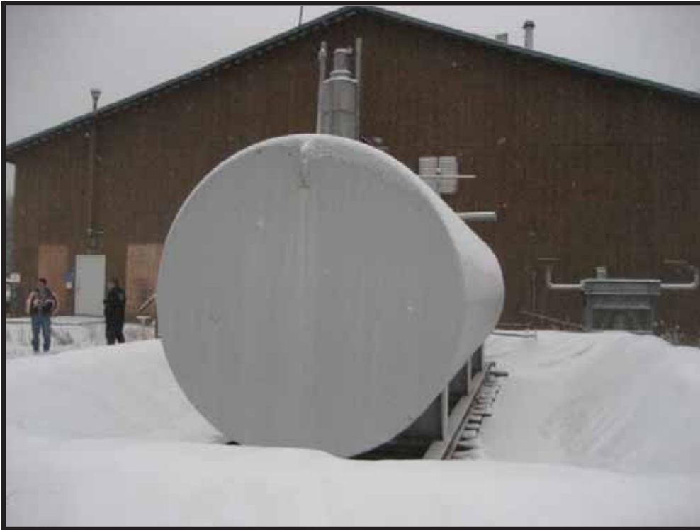
Photo 1: 10,000 gallon Generator Building AST with lined containment berm.
