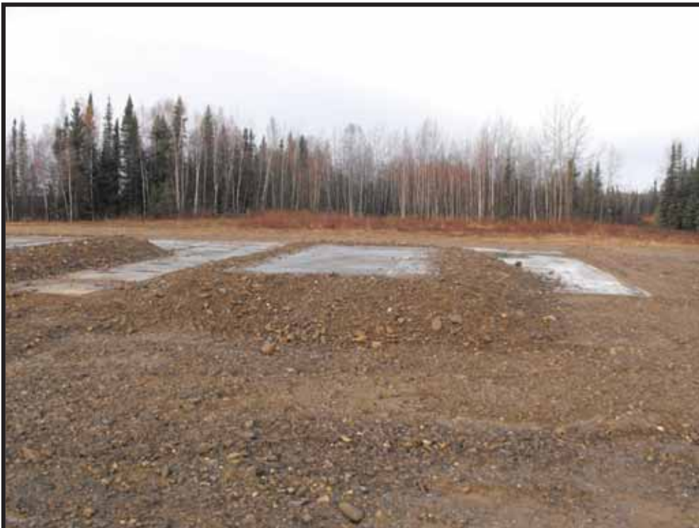
Photo 10: Looking west at north generator pedestal after surface cleaning with clean fill installed.
