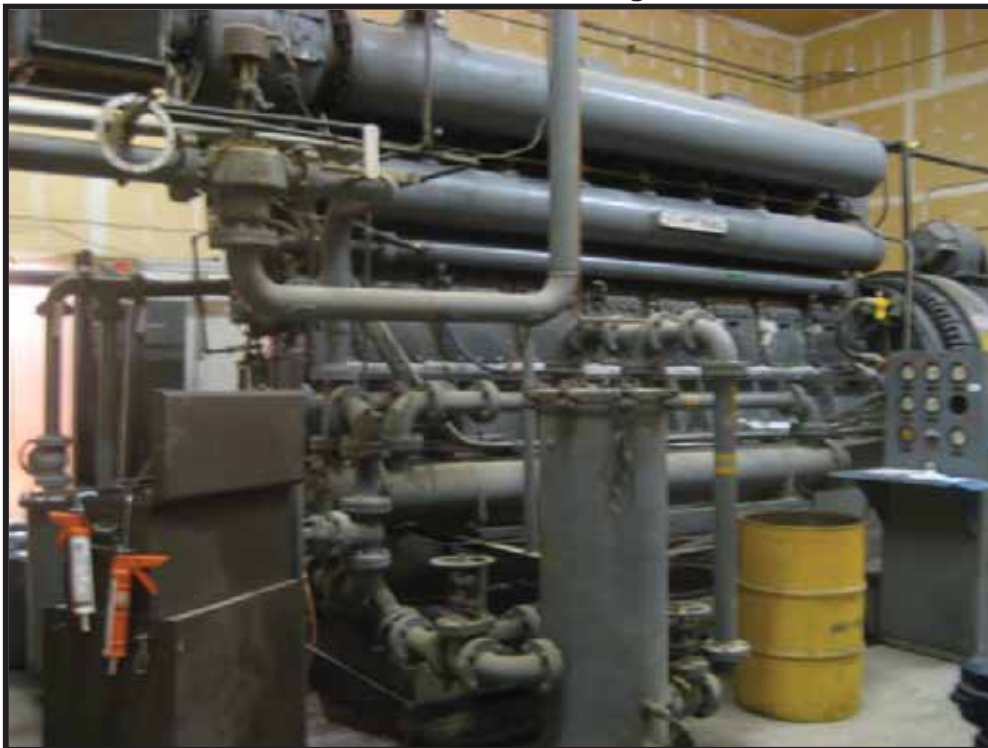
Photo 1: Looking southwest at one of two generators. Coolant system in foreground with fuel pump on left.
