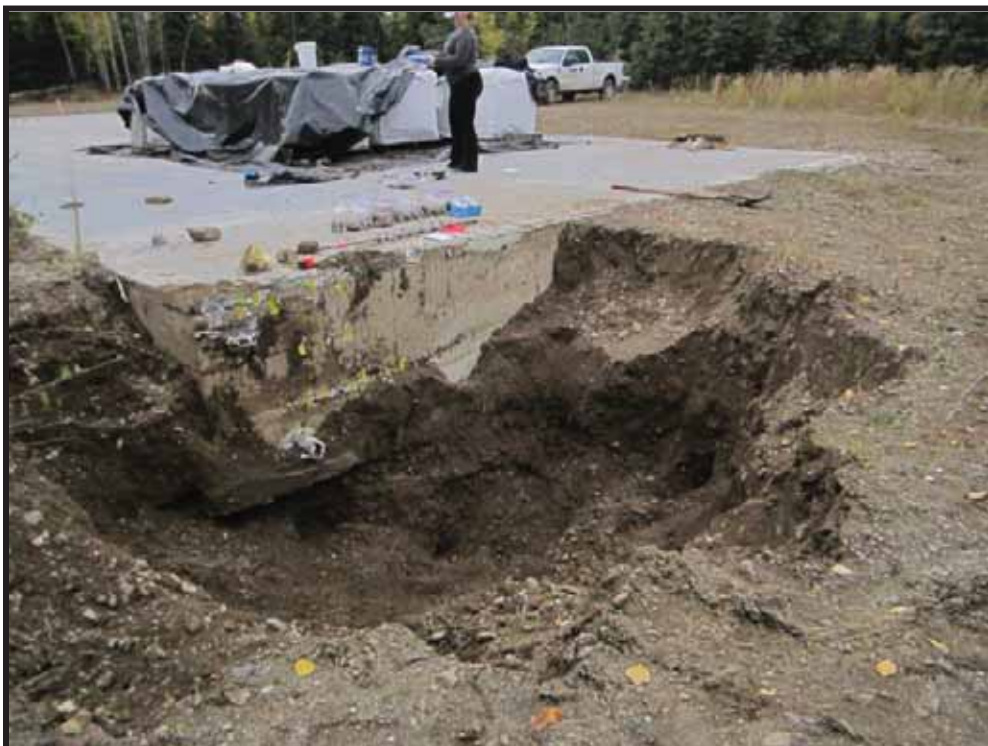
Photo 4: Looking southeast showing LIDAR AST excavation limits with containerized mercury-contaminated soil on slab.
