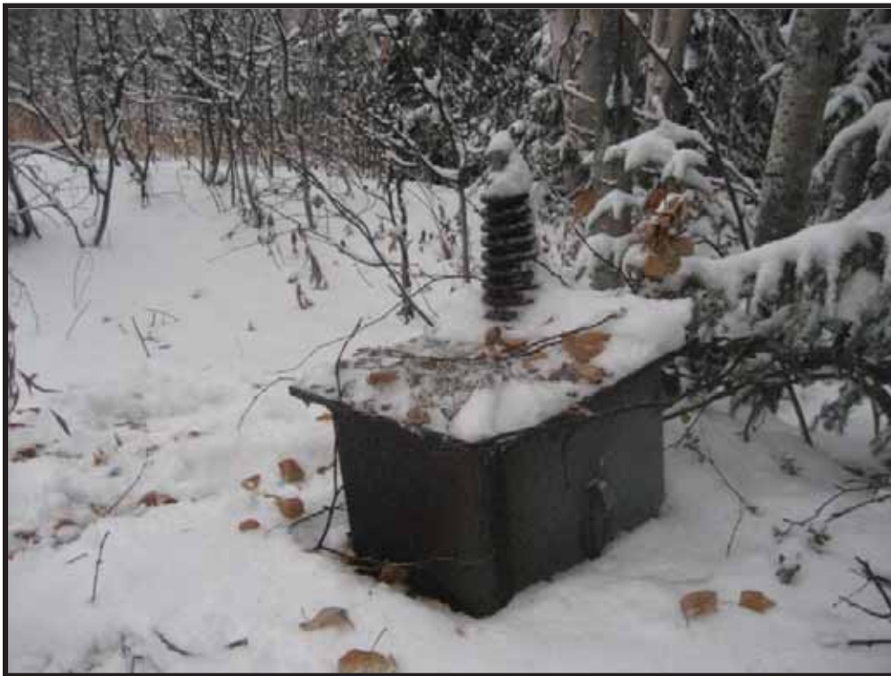
Photo 1: Abandoned transformer in the LIDAR area.
