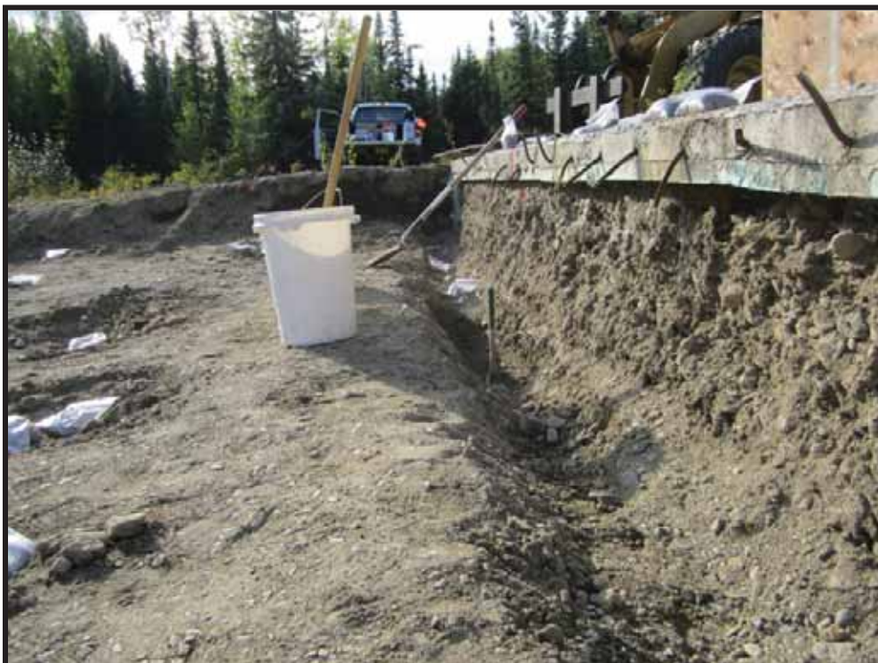
Photo 6: Typical hand excavation of soil and debris beneath LIDAR Tower with field screening samples visible to left and right.
