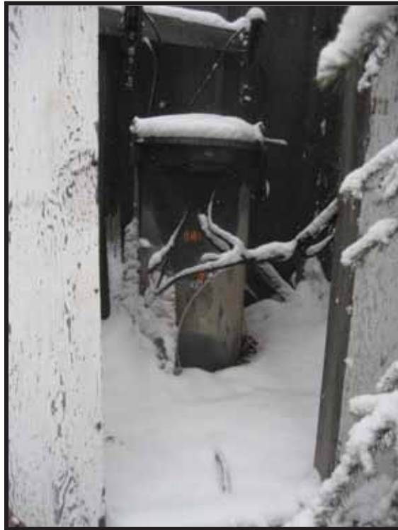
Photo 1: The Boneyard area transformer and shed.
