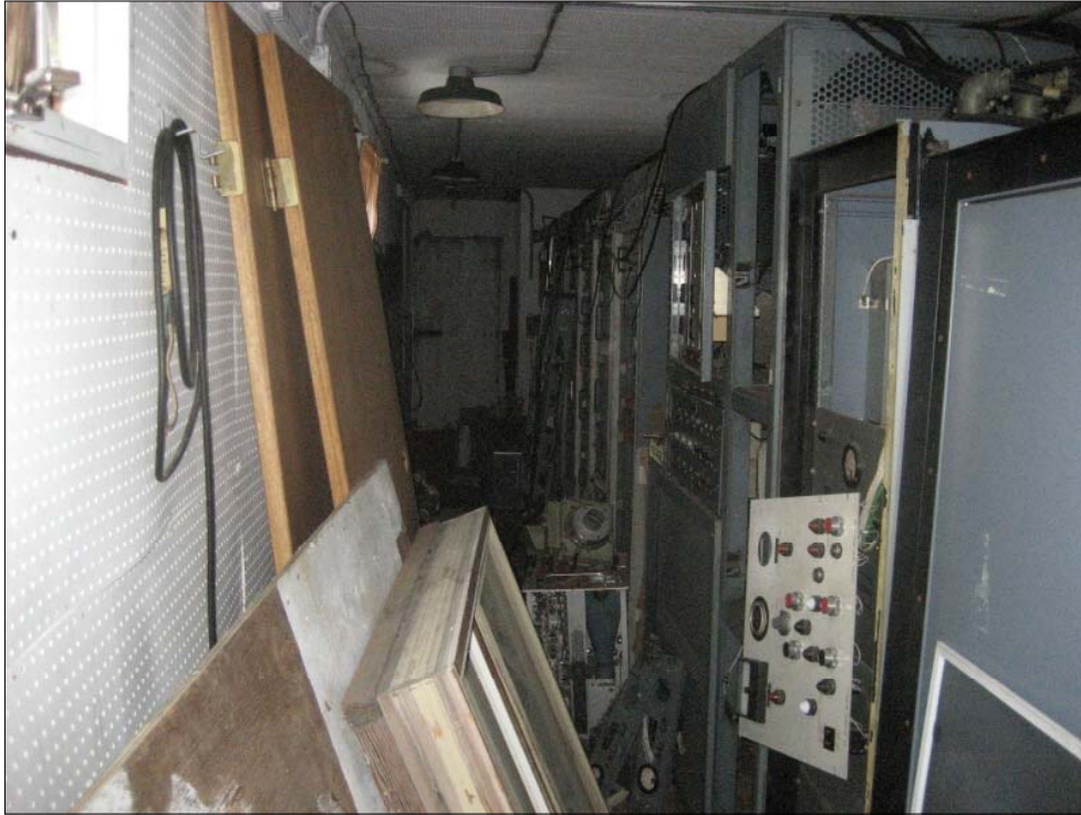
Photo 17 - Old electronic equipment inside the trailer structures located in the boneyard and believed to have been used by the Chena Valley Radio facility in conjunction with the collapsed dish nearby
