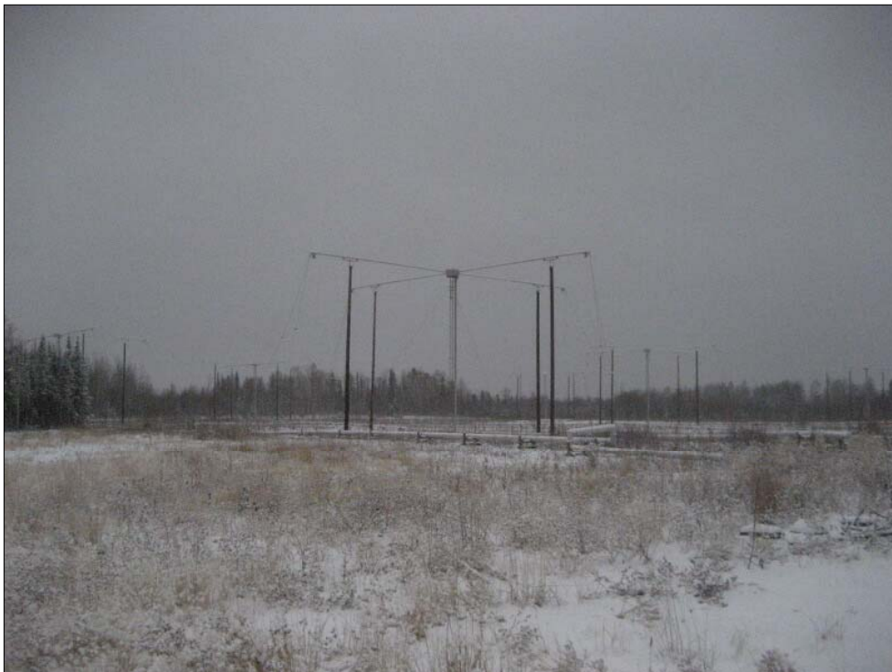
Photo 12 - Primary circular antenna array northeast of the Transmitter Building
