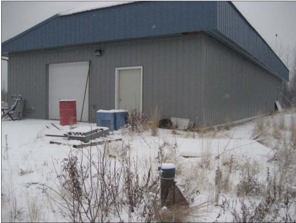
Photo 11 - North and west sides of transmitter building with water supply well in foreground and drum of used dielectric oil near overhead door
