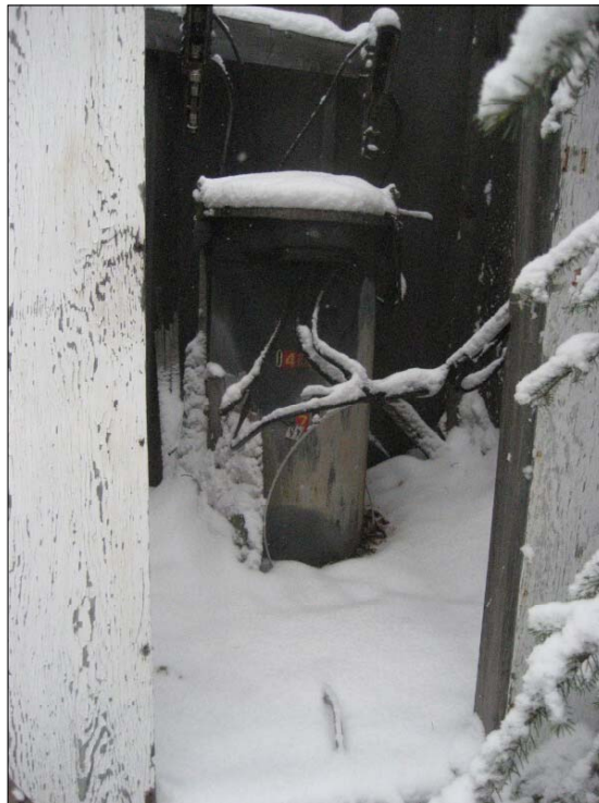
Photo 18 - Exterior electrical transformer believed to have powered the equipment in the Chena Valley Radio trailers in the boneyard (this unit is not believed to be powered currently)
