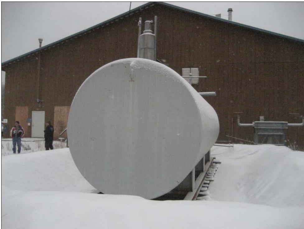
Photo 04 - 10,000 gallon diesel/heating oil storage tank in secondary containment on east side of Generator Building that supplies fuel to the generators and furnaces in both the Generator and Transmitter Buildings
