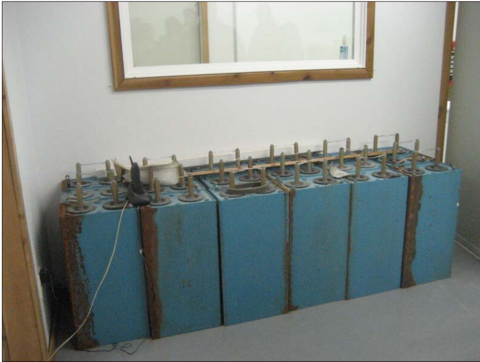
Photo 25 - Typical capacitors stored inside the LIDAR Building; similar capacitors also installed or stored in most other buildings
