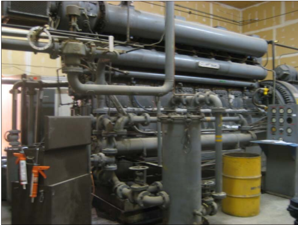
Photo 01 - One of two generators inside generator building; both appear well maintained with minimal staining around the oil and glycol (yellow drum) filters and reservoirs
