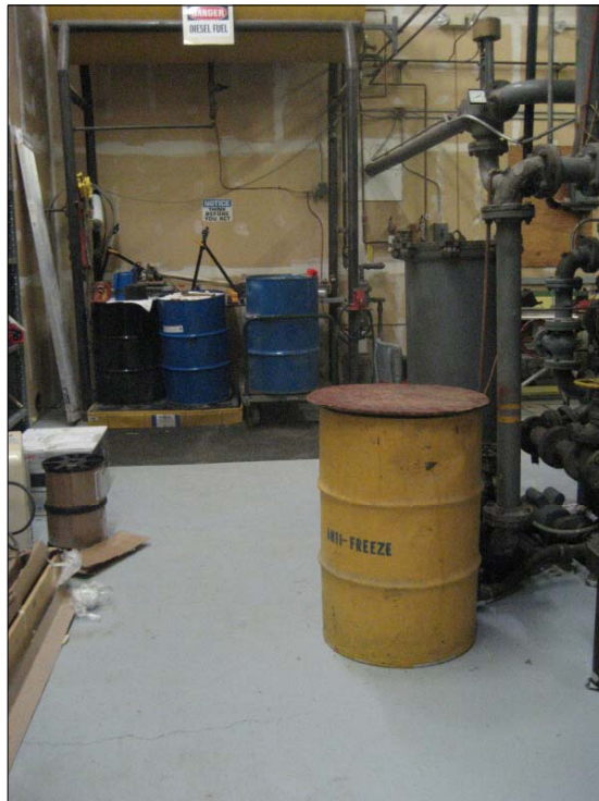
Photo 02 - Oil and coolant storage inside generator building: coolant overflow from generator in foreground, used and new coolant and oil in drums on spill pallet, and fuel storage "day tank" above drums
