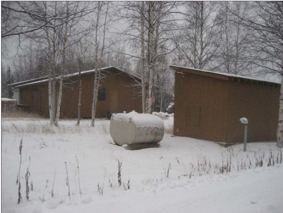
Photo 32 - Looking north the emergency generator building (foreground right) and associated fuel storage tank with at the Bunkhouse in the background
