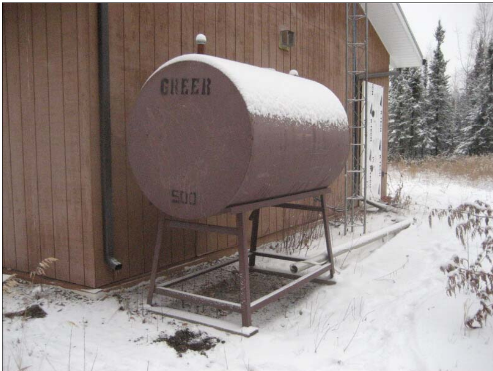
Photo 20 -Heating oil storage tank near northeast corner of LIDAR Building, which was reportedly overfilled but has not been reported to ADEC
