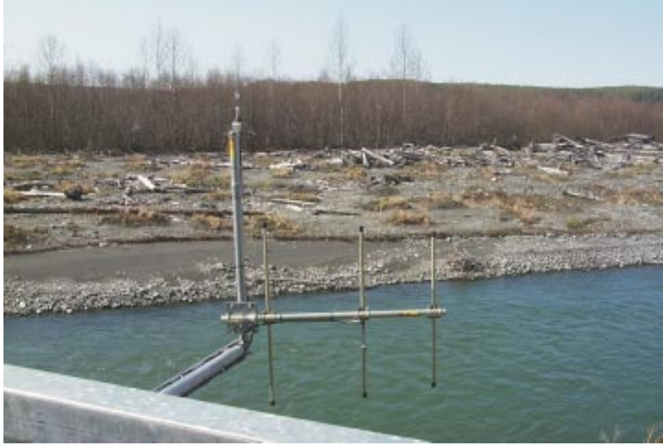
Figure III-5-6. Base station antennas.
