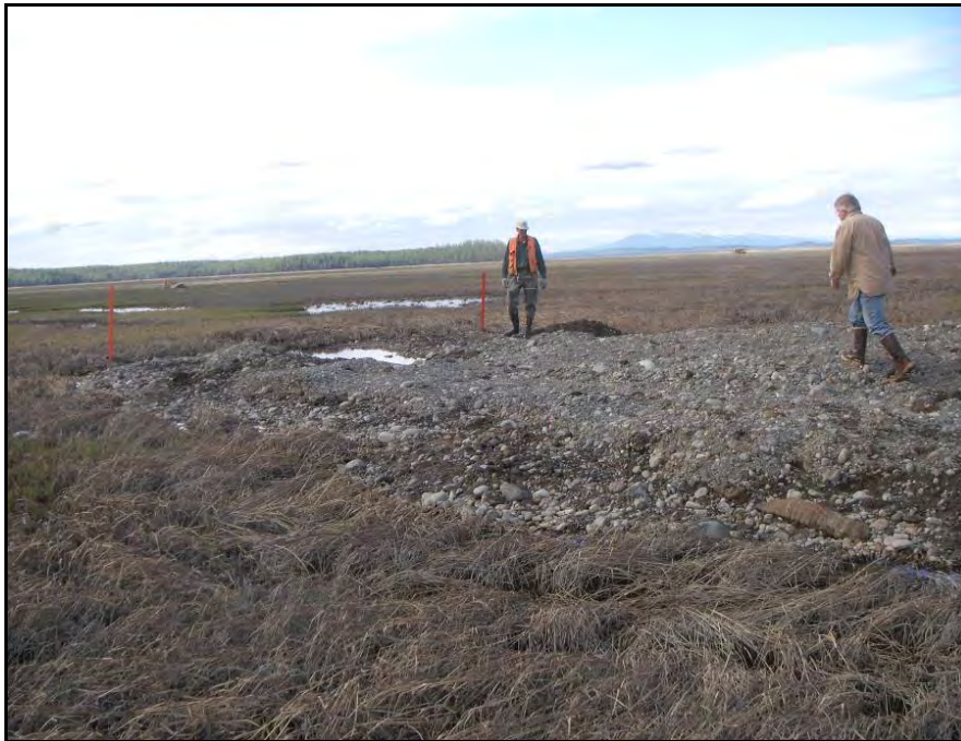
b. View from ground level looking northwest (Spring). Figure III-1-4. Capped pond following the first winter.
