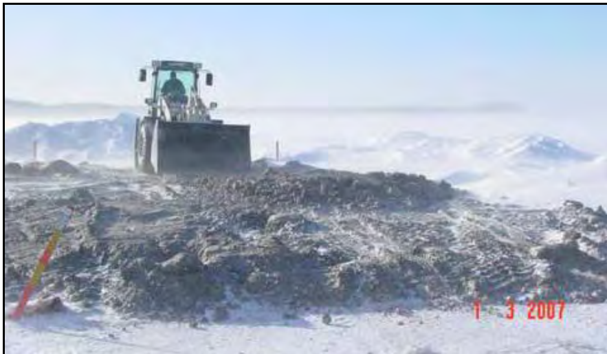
b. Spreading last load of gravel. Wind and drifting snow are evident. Figure III-1-3. Winter capping operations on Pond 23.
