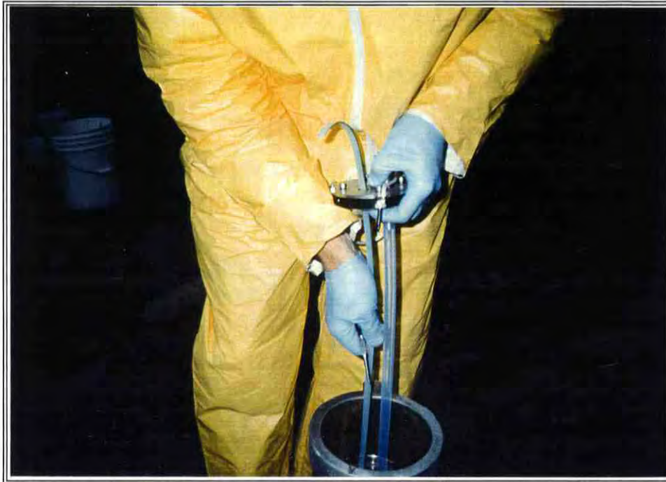
PHOTO 15: The power cable is being pulled through the well cap. A connector will be wired to the end of the cable for quick connection while sampling.
