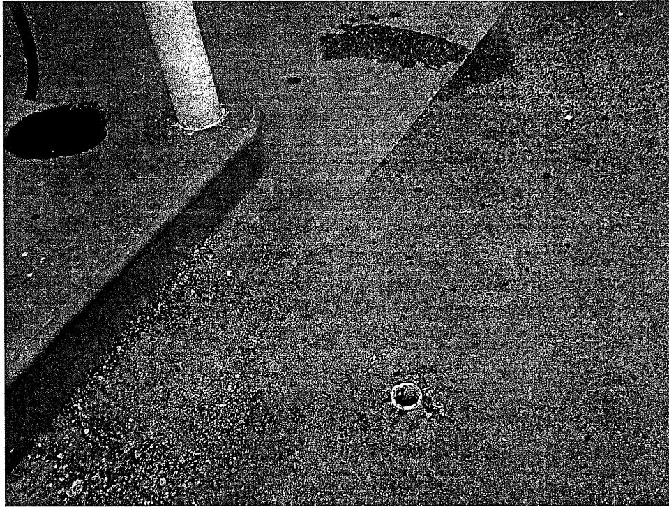
Old well casing (1994 installation) under influence of island run-off (MW-23)
