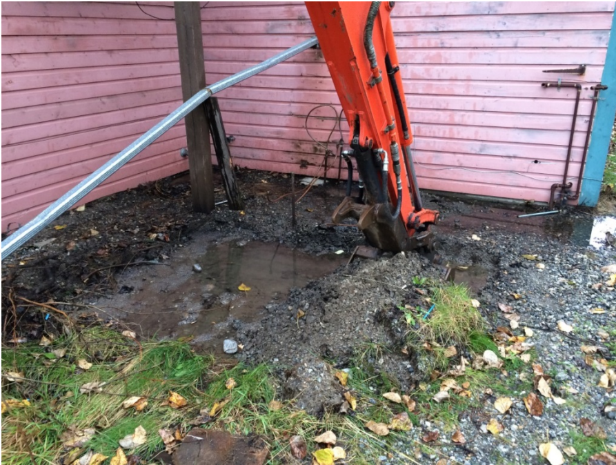
Photograph 3 – “hot spot” area directly below the former ASTs (looking north) showing dark grey surficial staining.
