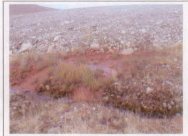
Photo 6-5: Large seep area near creek on the southeast side of the Landfill Cap.
