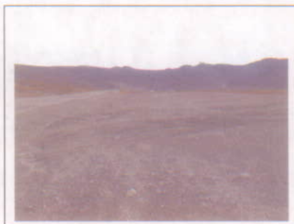
Photo 6-3: Tire track ruts at north side of the cap near the road.
