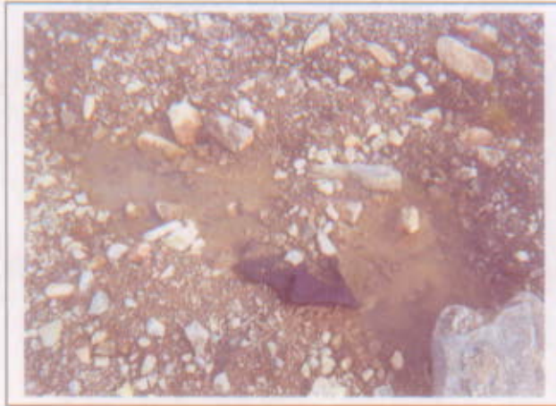
Photo 6-4: Exposed liner on southeast slope of Landfill Cap.
