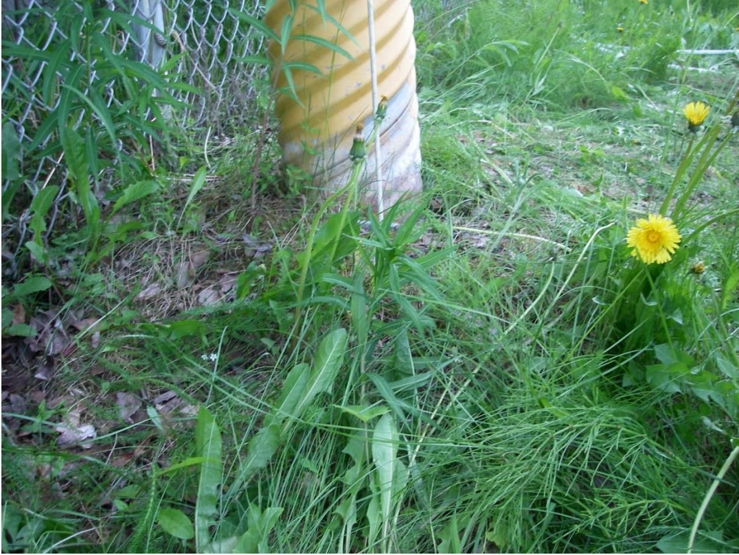
Photo 9: AP-3231 uplift around base of well
