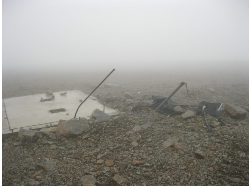
Photo No. 34 – 21 August 2012 SS015 UST Spill Area; Concrete foundation at southeast end of site; view facing east.
