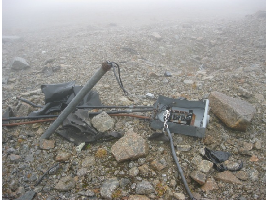
Photo No. 35 – 21 August 2012 SS015 UST Spill Area; Electrical components of foundation.
