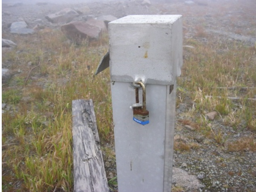
Photo No. 33 – 21 August 2012 SS015 UST Spill Area; WW03; view facing north.
