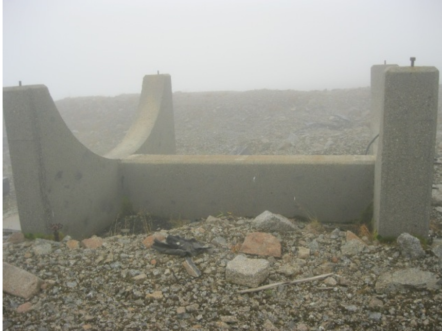
Photo No. 36 – 21 August 2012 SS015 UST Spill Area; AST cradle at southeast end of site; view facing west.
