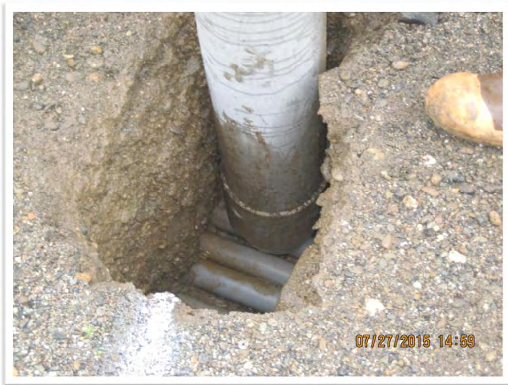
Photograph 3 – A vacuum truck (shown) was used to expose buried utilities prior to start of excavation work.
