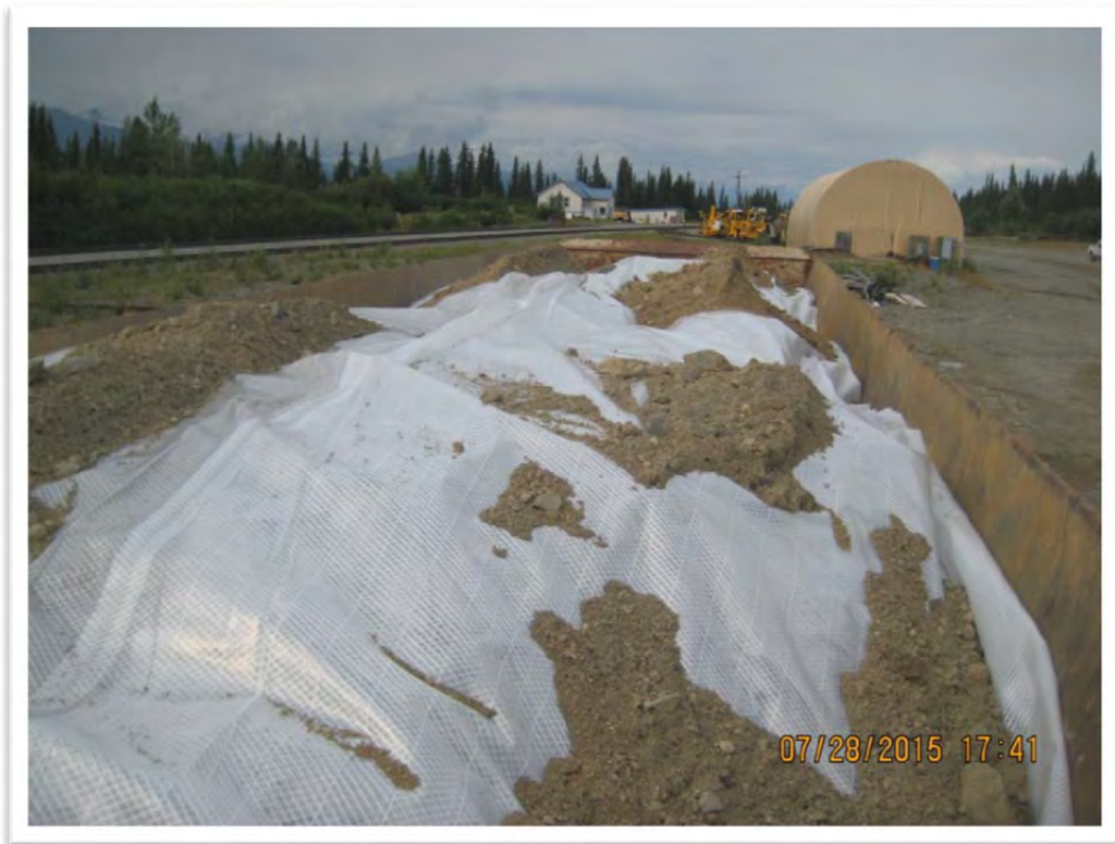
Photograph 12 – View of covered soil in one of the two railcars. Clean soil material was used to keep the plastic covers in place. View to north.
