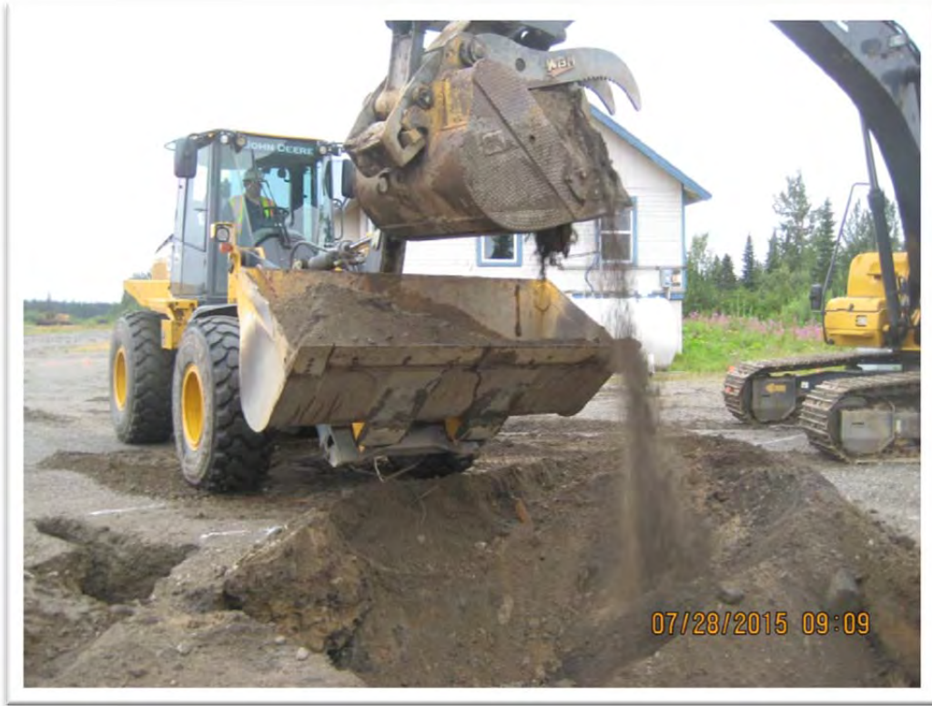
Photograph 5 – Excavated soil was loaded into the bucket and immediately placed in a railcar. View to southwest.
