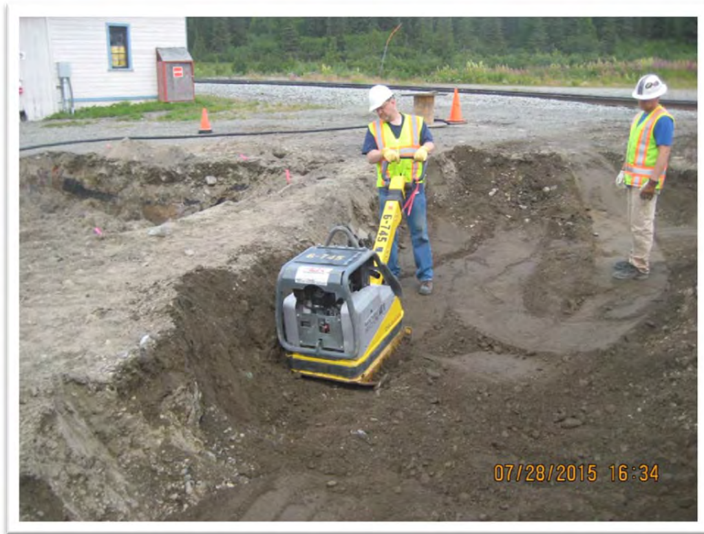
Photograph 9 – View of clean backfill being compacted in lifts in the South Excavation. The North Excavation and tool shed are in the left of the photograph. View to east.
