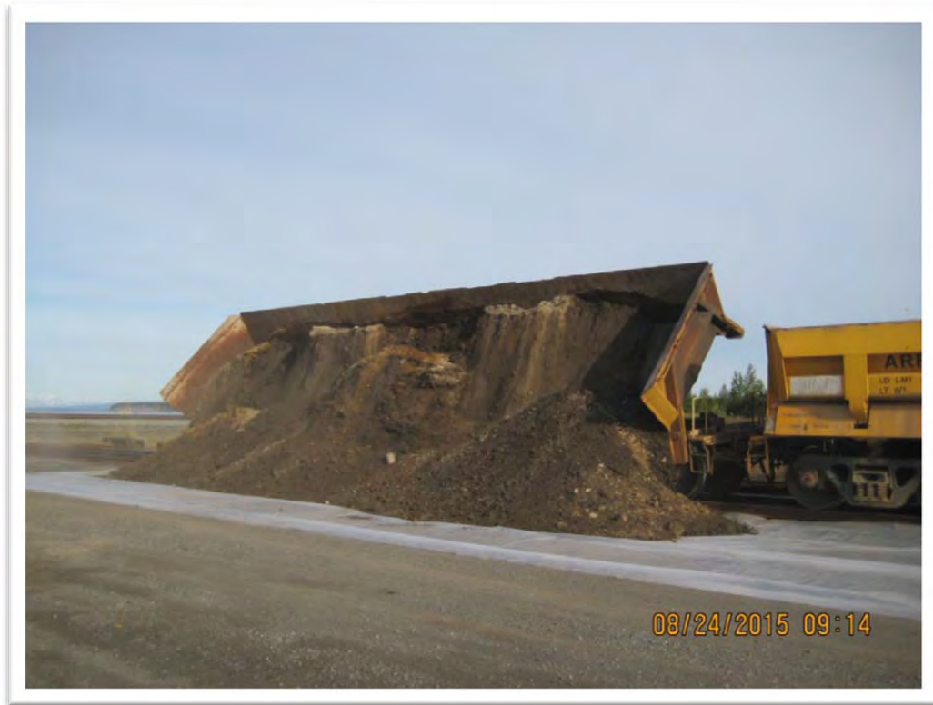
Photograph 13 – A total of 132 tons of contaminated soil was transferred from the Hurricane site to the Anchorage Yard using two side dump railcars. View to northwest.
