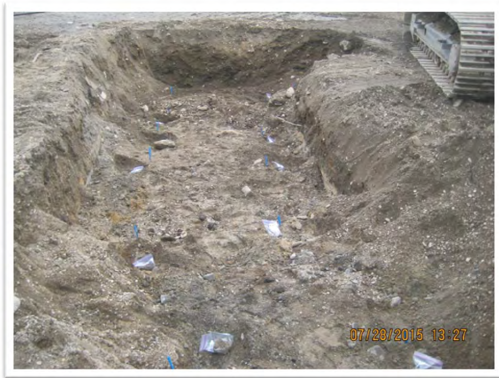
Photograph 7 – View of floor confirmation sample locations (represented by blue whiskers) and the limits of the South Excavation. View to east.
