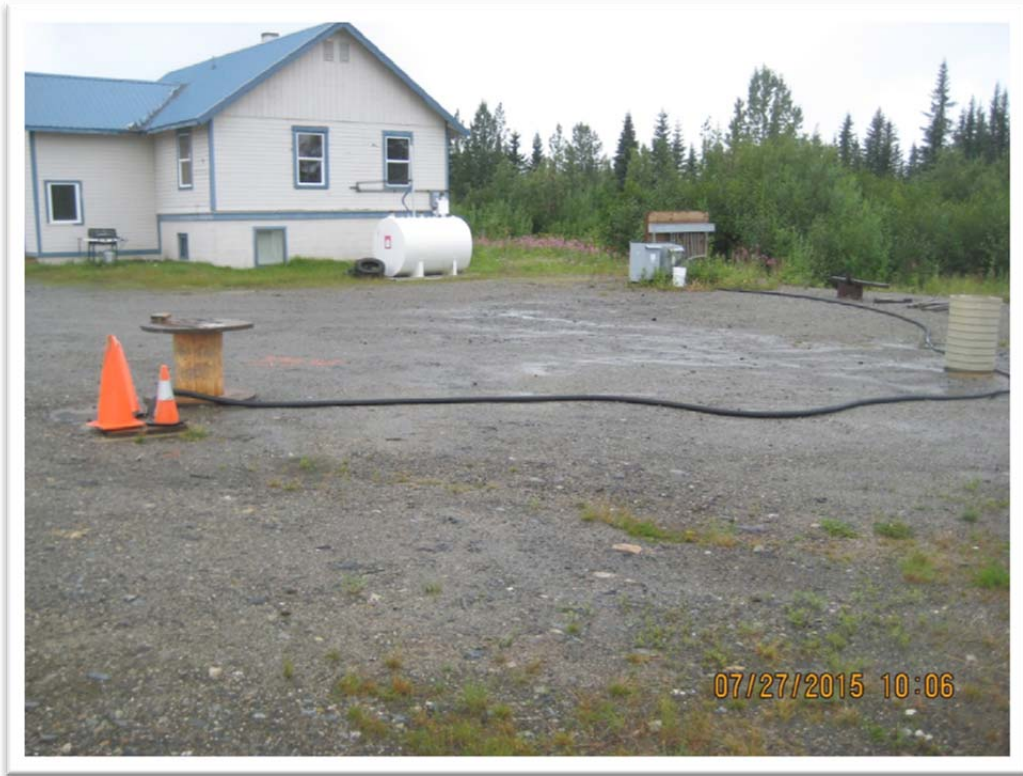
Photograph 1 – View of site prior to excavation with Hurricane Section House in background. View to west.
