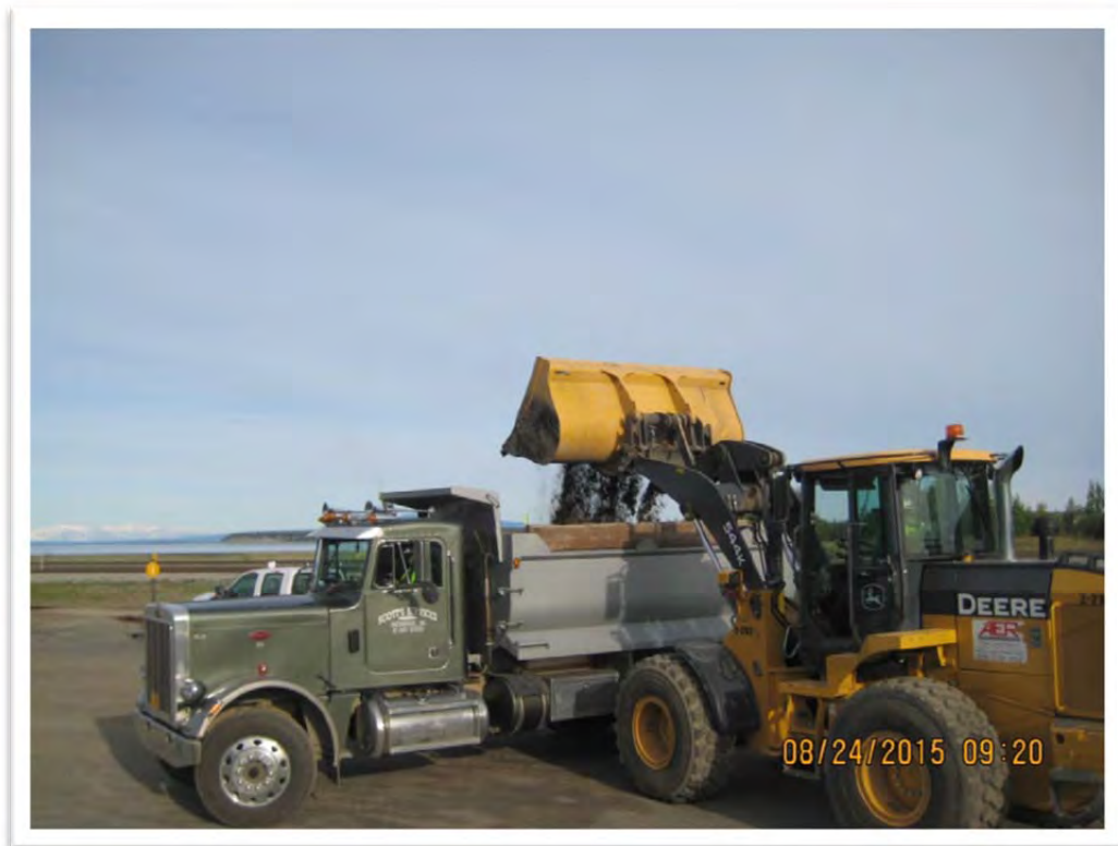
Photograph 14 – The contaminated soil was loaded into dump trucks and transferred from the Anchorage Yard to Alaska Soil Recycling for thermal treatment. View to northwest.
