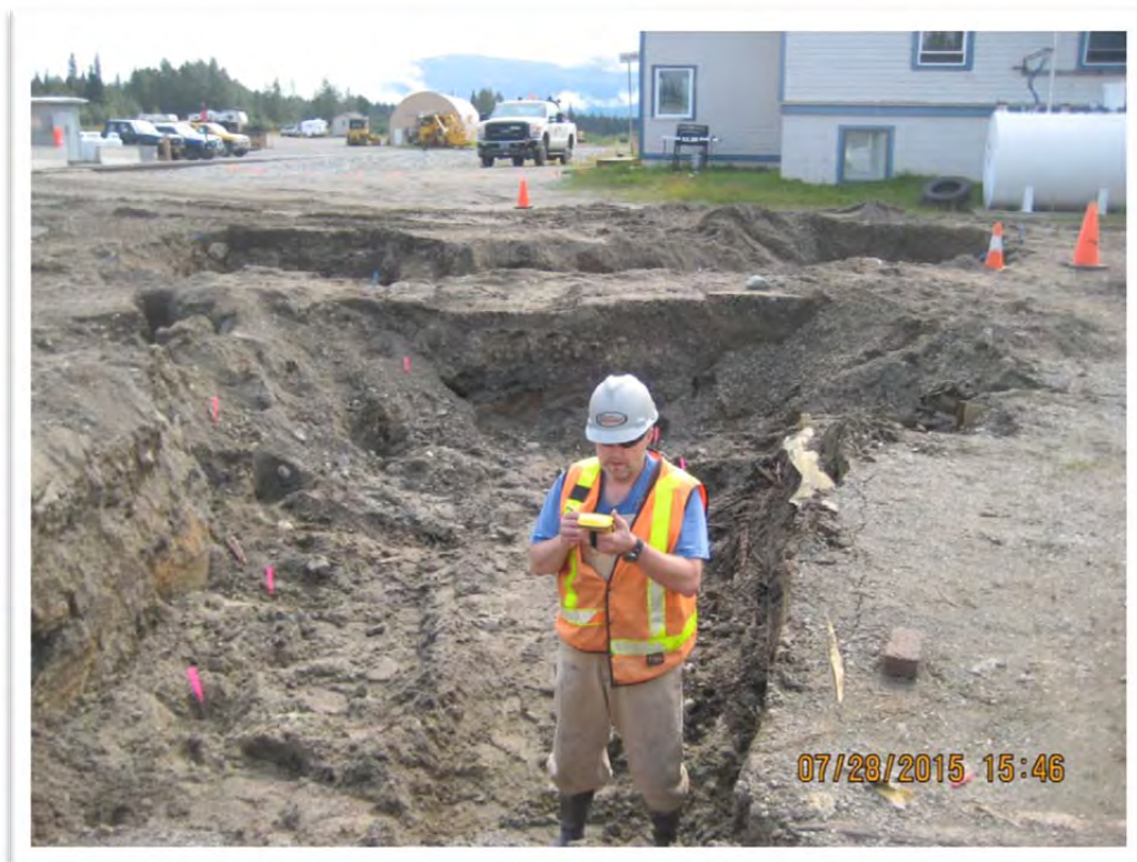
Photograph 8 – The locations of the excavation corners and confirmation samples were measured with a GPS. The North Excavation is in the foreground and the South Excavation is in the background. View to southwest.
