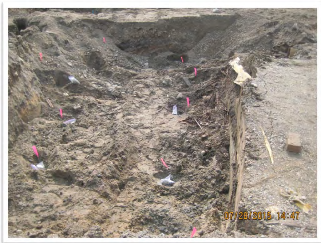
Photograph 6 – View of floor confirmation sample locations (represented by pink whiskers) and the limits of the North Excavation. Foundation is on the right of photograph. View to southwest.
