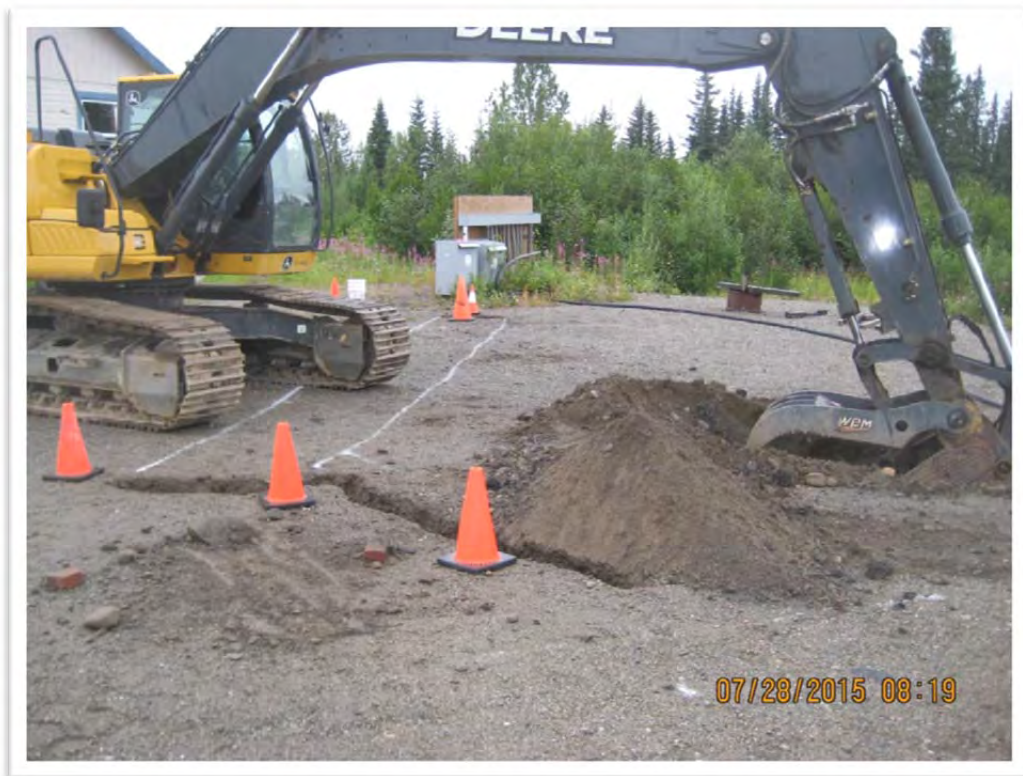
Photograph 4– This photograph shows the beginning of the North Excavation. This excavation was confined by buried utilities (shown in white paint and in the vacuum truck excavation) and a foundation (not shown). View to west.
