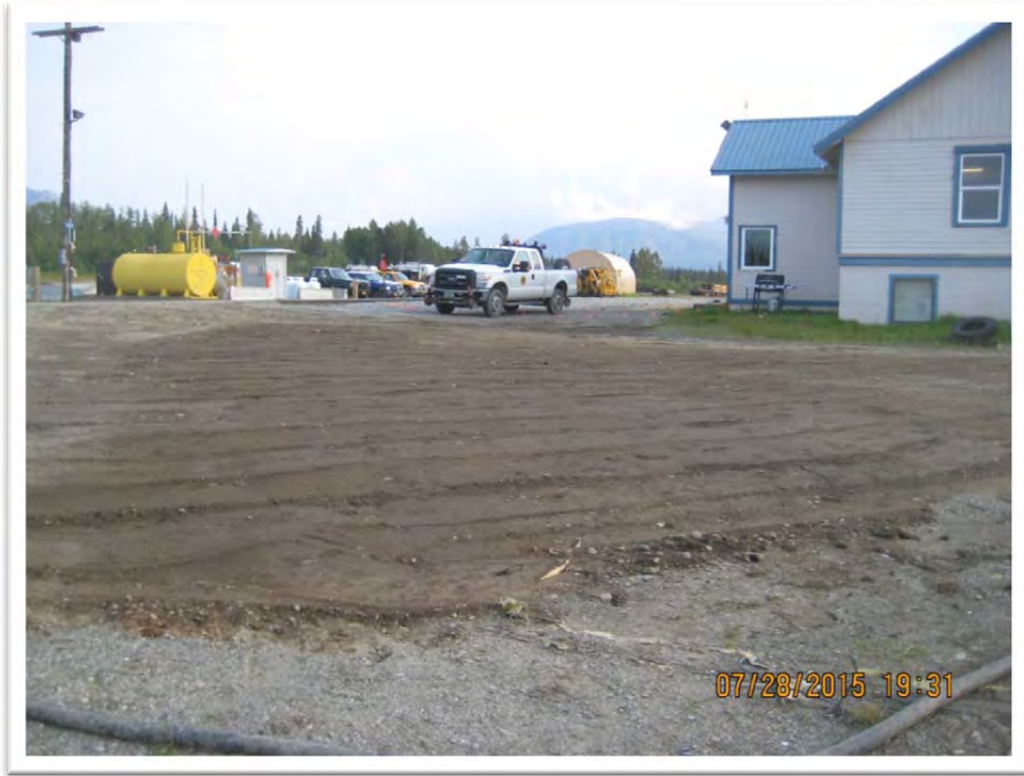
Photograph 11 – View of site after excavation work and backfill completed. View to south.
