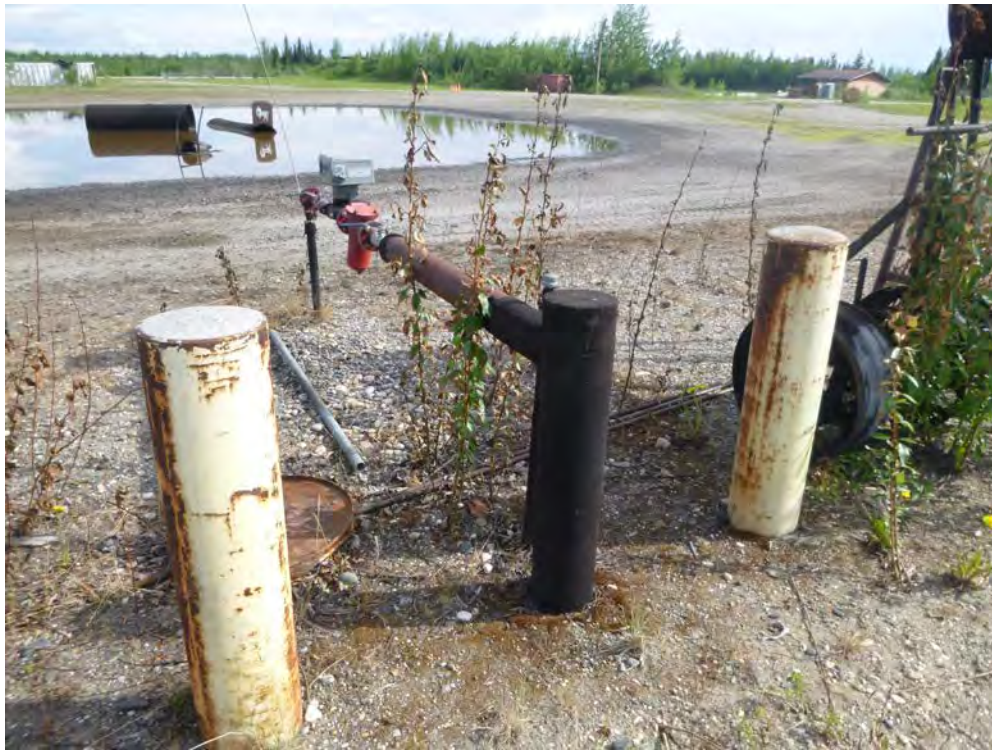
Photo 5: Fuel conveyance piping and flow meter to the north of the FTP pond (June 5, 2018).
