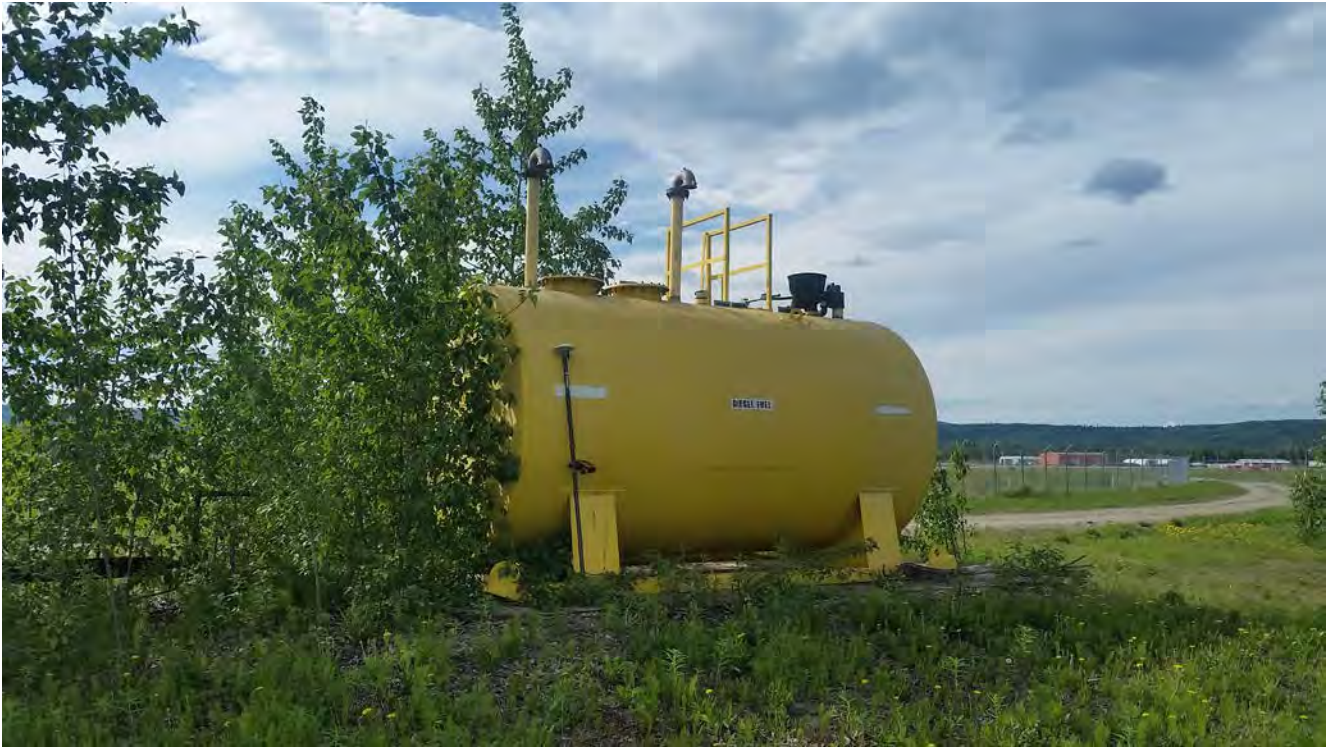
Photo 7: Diesel supply tank for FTP, view to north (June 5, 2018).
