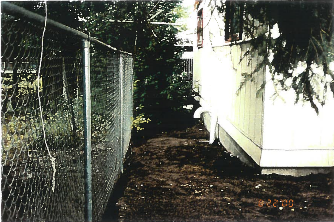
Photo 7: View of back of the house on August 22, 2000 after installation of intake vent and backfilling.
