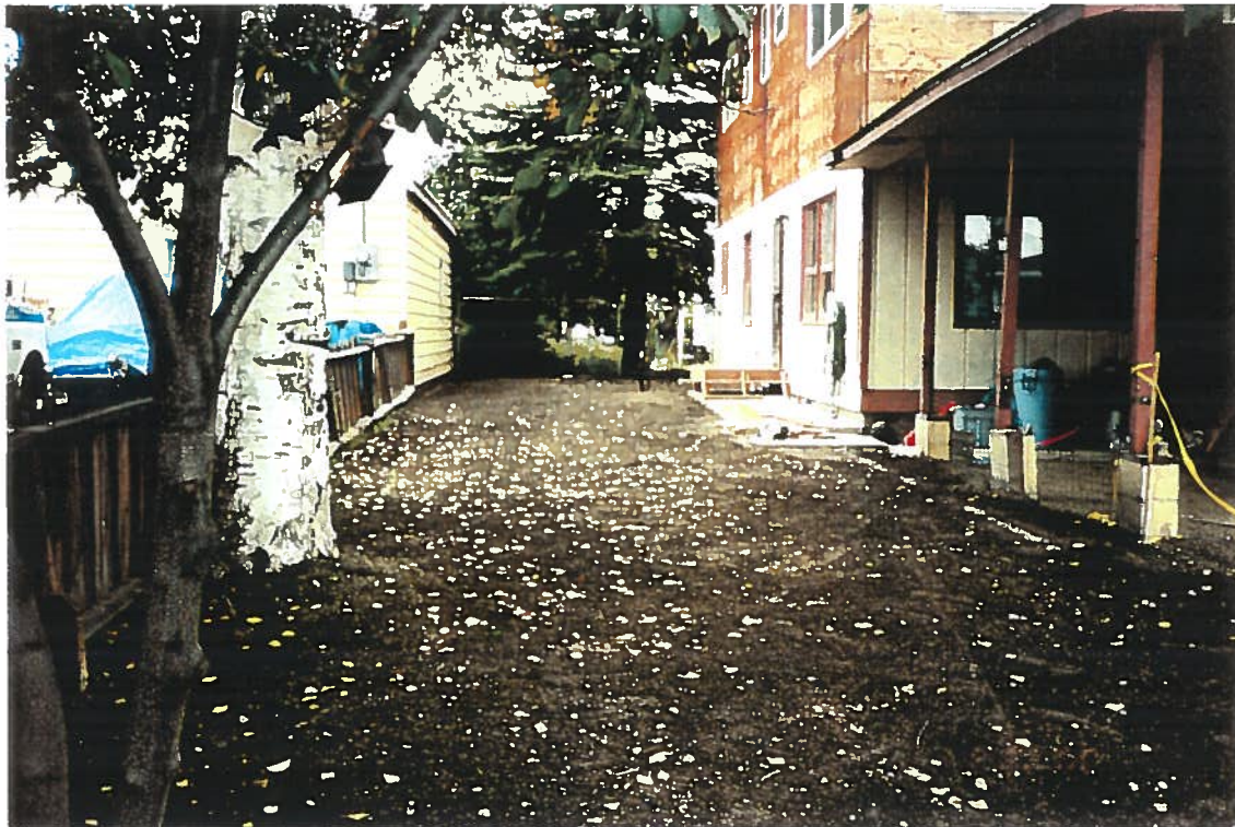
Photo 8: Appearance of site on August 22, 2000 after completion of landscaping and seeding. To the side of the house is the new sidewalk and porch.
