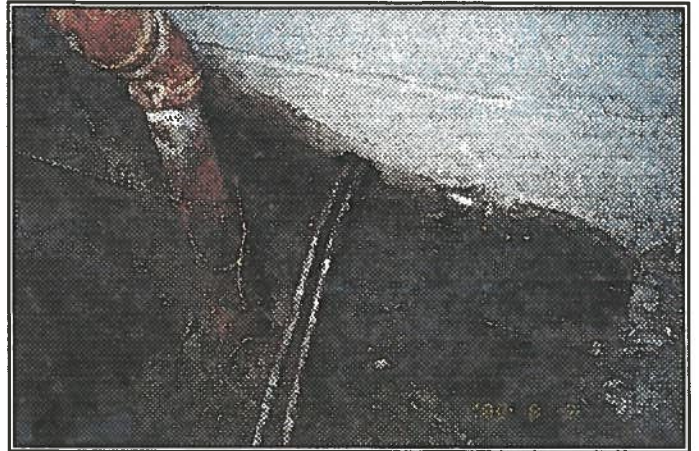
Vent Pipe for UST, 8/2/00. Fuel Lines going through foundation wall.
