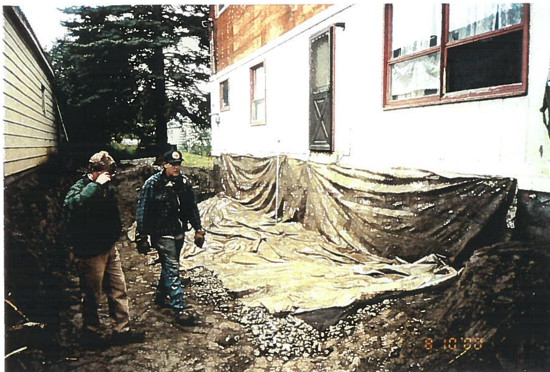
Photo 4: Installation on August 10, 2000 of the plastic and liner overlying the intake pipe for the vapor recovery system
