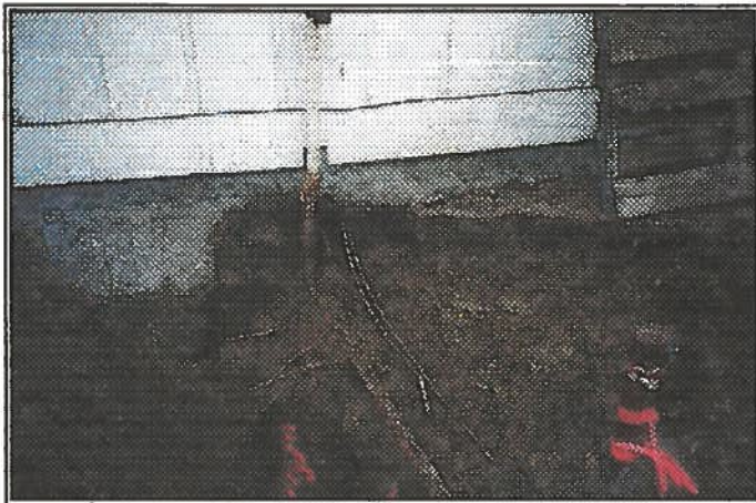
Lines & vent pipe, 8/3/00.
