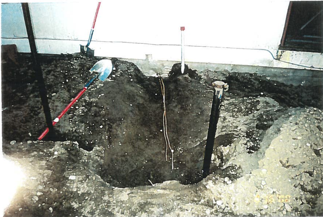
Photo 6: Close up view of installation of the new underground storage tank and fuel lines.
