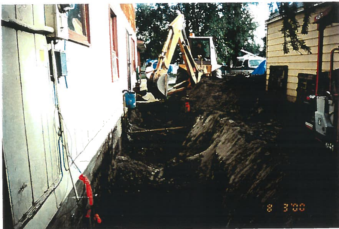
Photo 3: Looking north on August 3, 2000 at excavation in the vicinity of the former underground storage tank.
