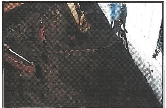
Another view of fuel lines & vent pipe. Excavating contaminated soil from area on 8/3/00.
