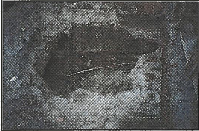
Fuel lines that were broken & repaired on 12/10/00, by I.C.C. Photo date 8/1/00 shows no significant staining from any leaks in the pit, showing fuel line repair.
