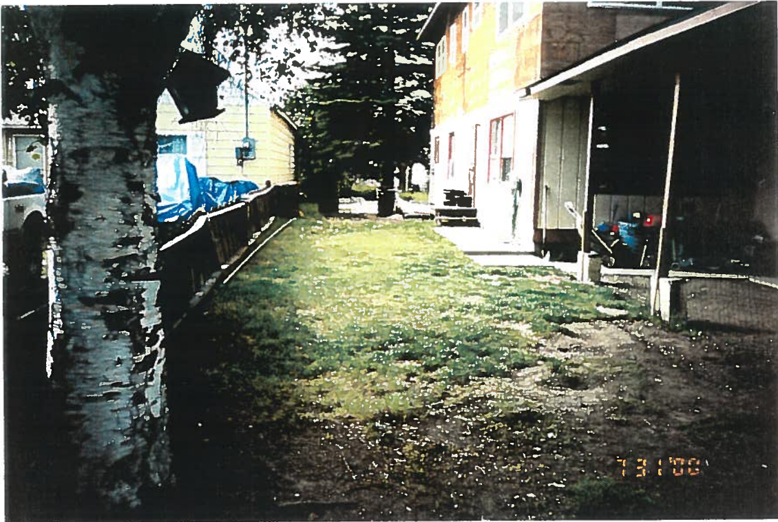
Photo 1: Appearance of site looking south on July 31, 2000 before excavation and removal of contaminated material. Drums in the background contain soil from previous investigation.
