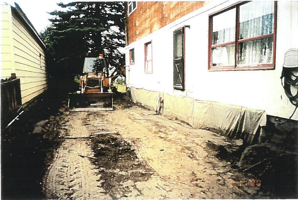
Photo 5: View of backfilling on August 11, 2000. Pipe near the side door of the house is monitoring well #1.
