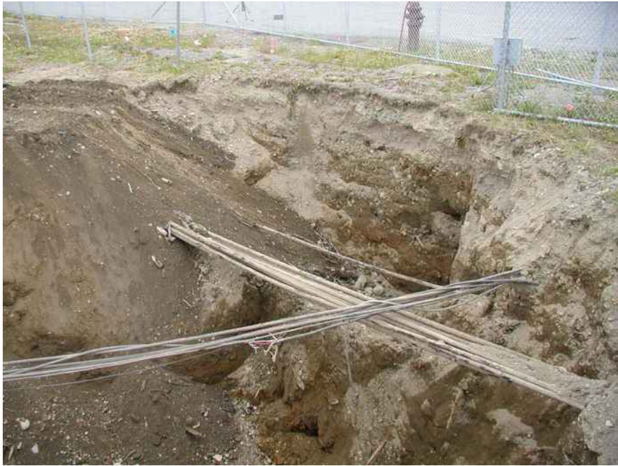
Photo 5. Exposed cables in open exvacation.
