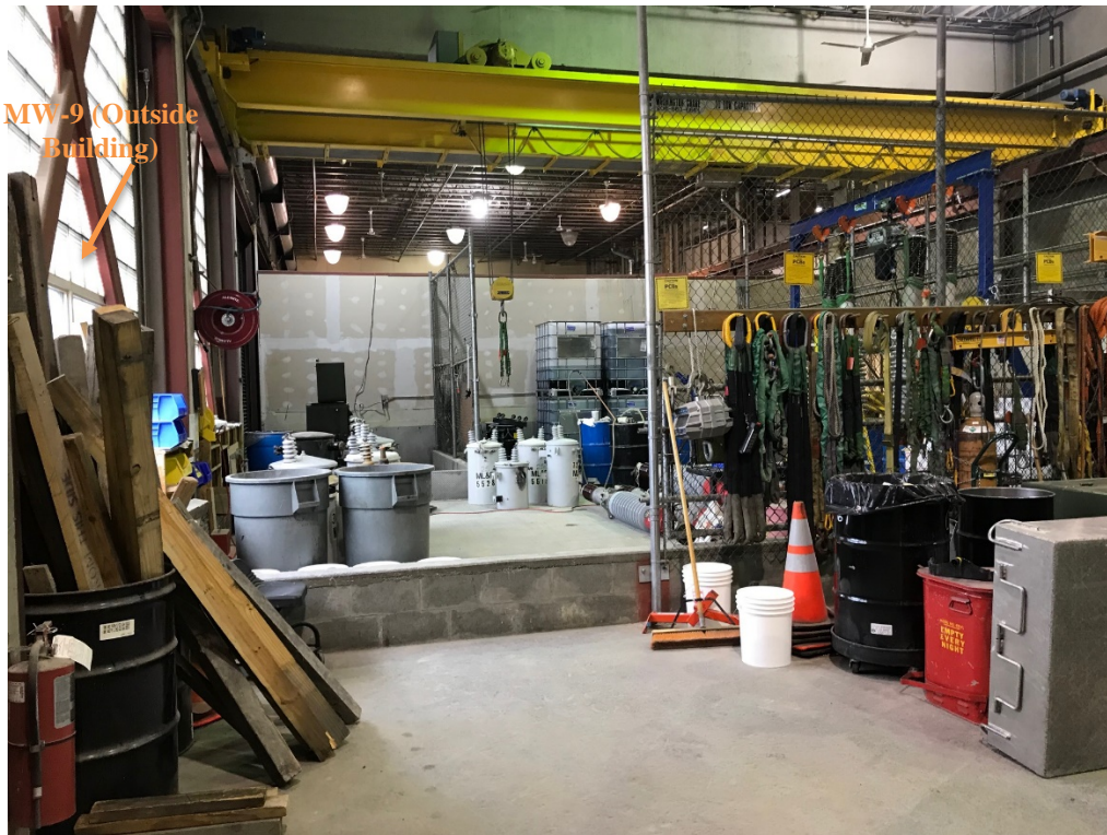
Photo 5: Inside of the Transformer Shop looking west into the Control Pit (Containment Area). MW-9 is located outside of the building, near the window on the left.
