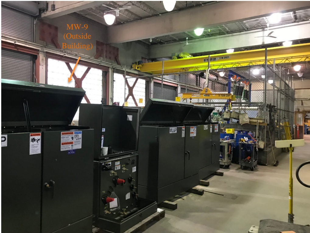
Photo 3: Inside of the Transformer Shop looking southwest. MW-9 is located just outside of the window on the left.
