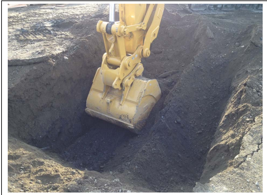
Photo 1: Looking southeast while excavating potentially contaminated soil at the TP-3/B-3 excavation. (October 24, 2014)
