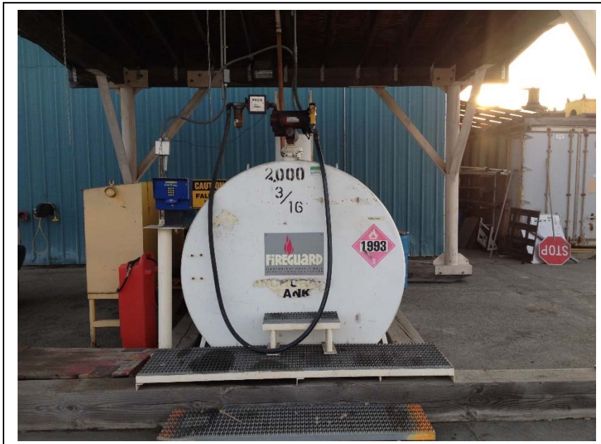
Photo 4: This 2,000-gallon, diesel, aboveground storage tank fueling facility was formerly located at the northwest corner of the proposed New Marine Storage Building. (October 24, 2014)
