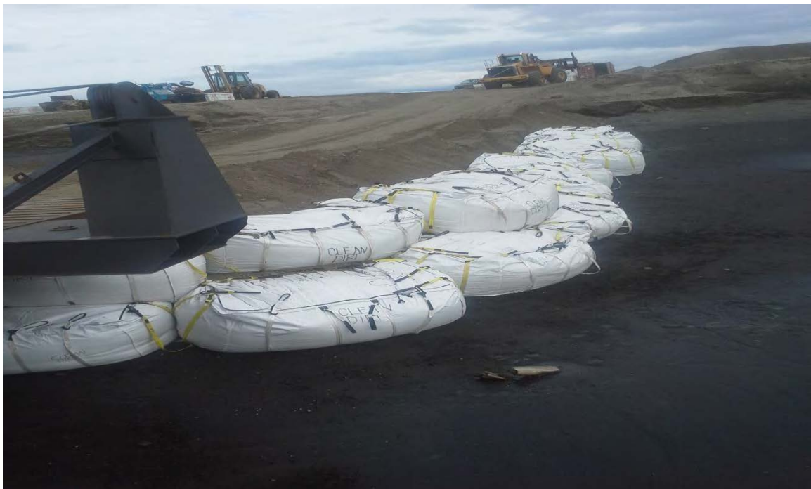
Photo 18: 10-CY super sacks filled with clean soil used to prevent ramp erosion, 2013
