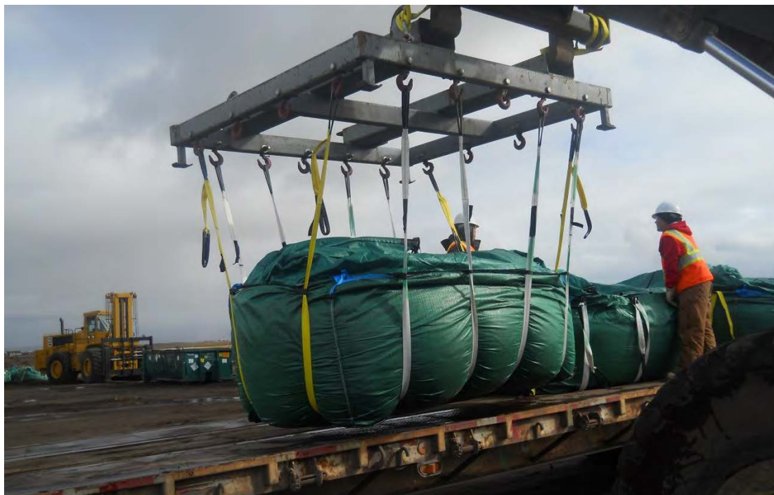
Photo 10: Loading low-boy trailer with 5-CY super sacks for transport to the barge, 2011
