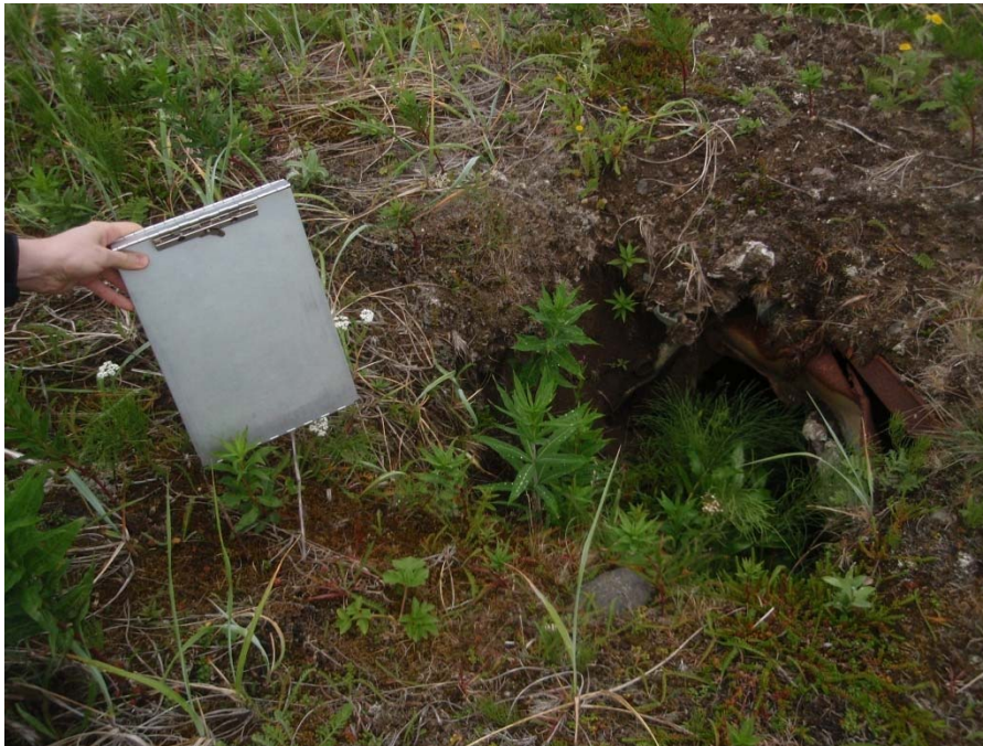
Photograph 10: LF007. North side facing downward toward subsidence with exposed debris.
