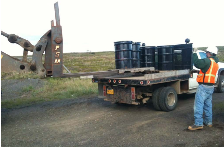
Photo No. 2 – 10 September 2014 Loading purge water and wastewater drums onto a flatbed truck. Looking north.
