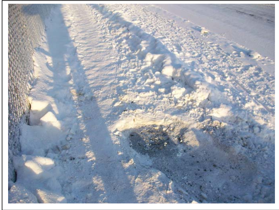
Photograph 3: Following the decommissioning of Monitoring Well MW4, the top 2 feet of the space created by removal of the monument was filled with gravel. The ground was resurfaced with cold patch asphalt to match surrounding conditions (December 18, 2009).
