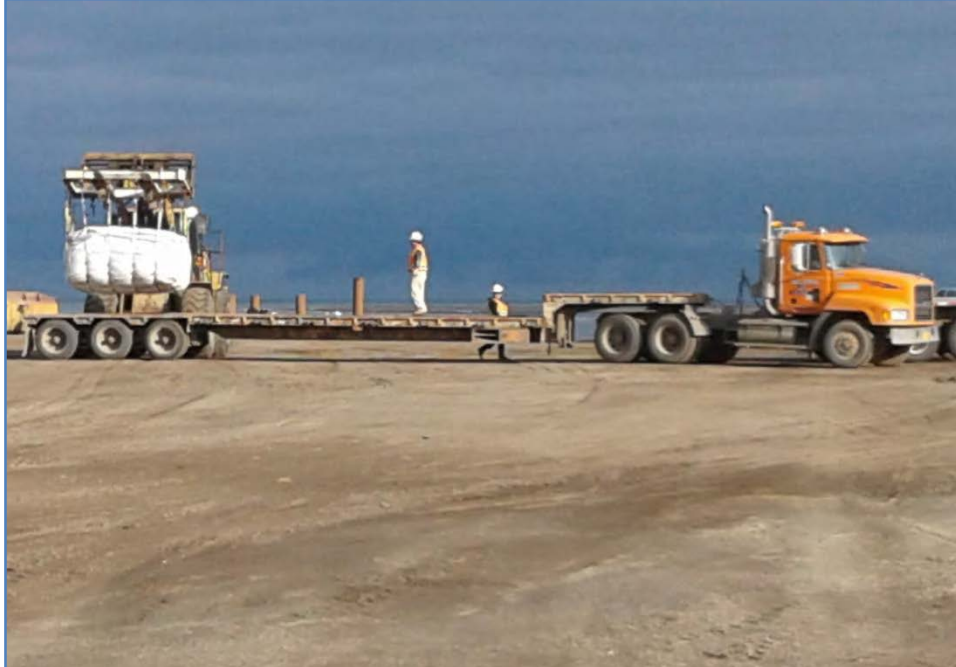
Photo No. 11 – 19 August 2016 Loading bags onto flatbed for waste transport. View facing northwest.
