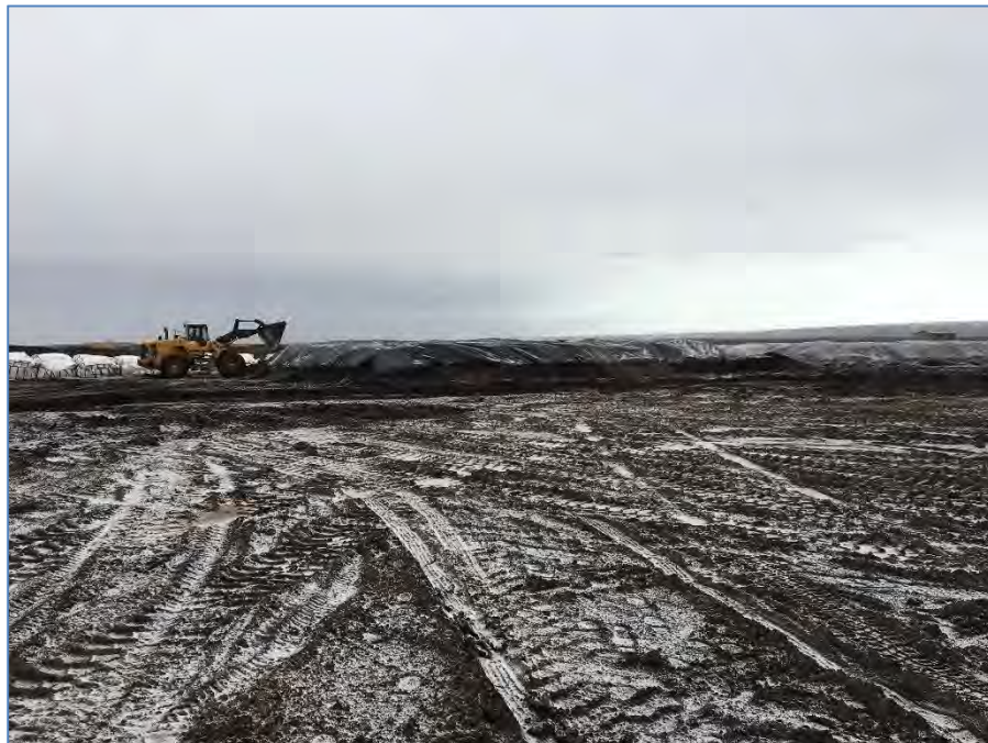
Photo No. 12 – 23 February 2018 Repairing top cover over the super sacks after winter storm. View looking northeast.
