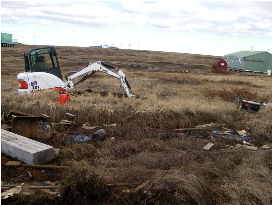
PHOTO 8: DIGGING TP-6 OUTSIDE OF BERM AT SOUTHEASTERN CORNER OF SITE; VIEW TO THE SOUTHEAST.
