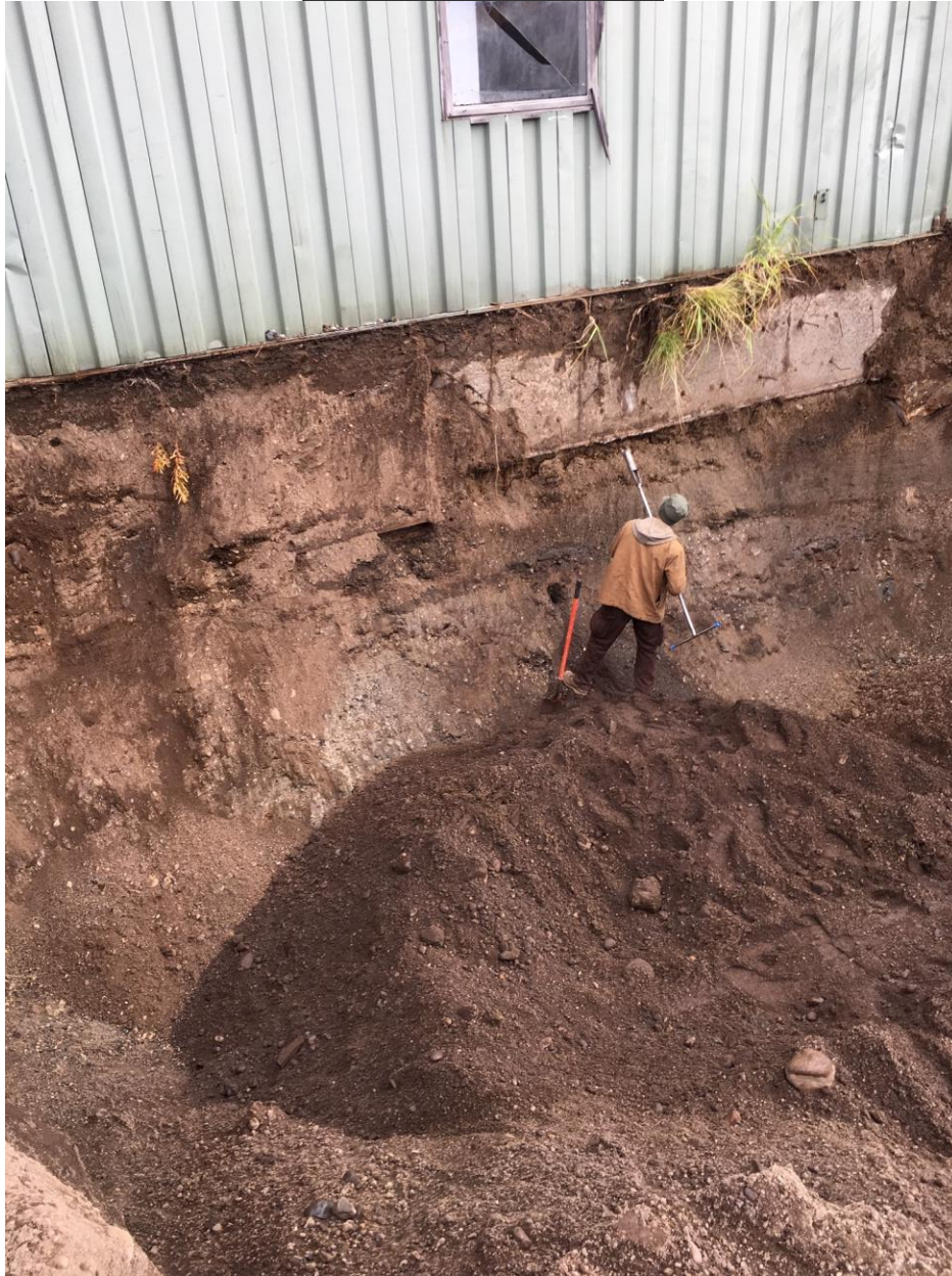
Photo 1: Beginning sample collection beneath the building footer. There is a visible lense of impacted material at the technician's waist level
