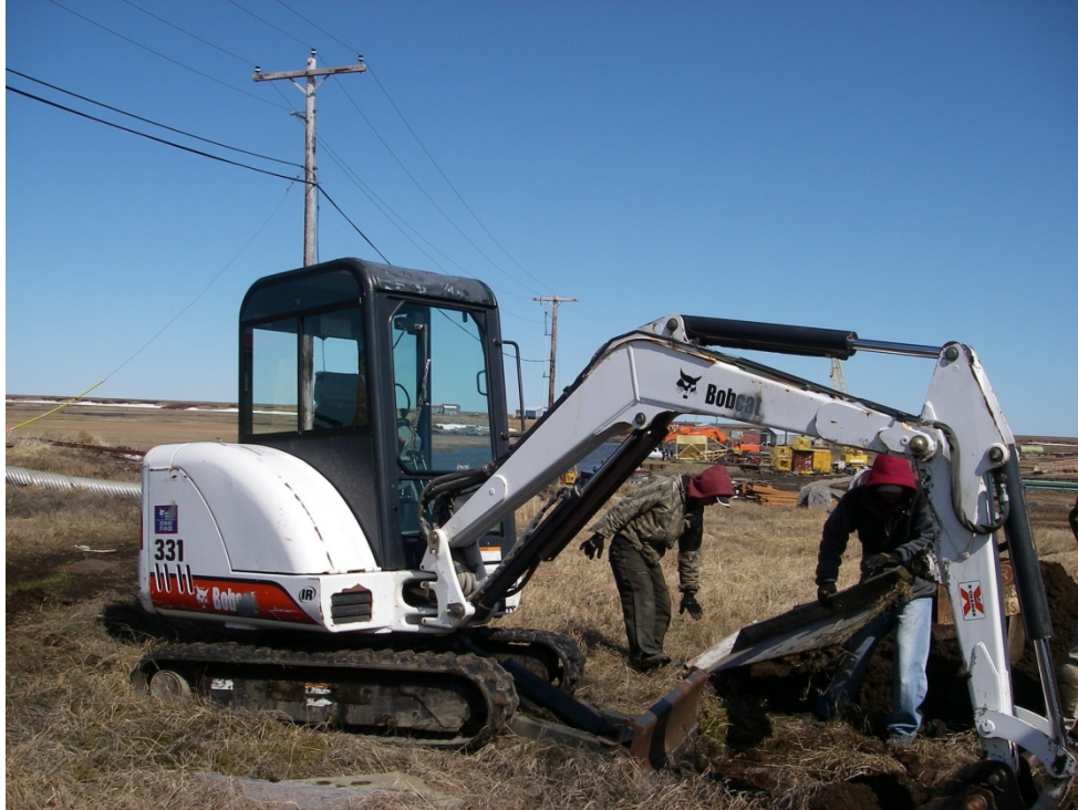
PHOTO 1: BACKHOE, OPERATOR, AND LABORER REMOVING DEBRIS BEFORE DIGGING TEST PIT TP-1, VIEW TO THE NORTH
