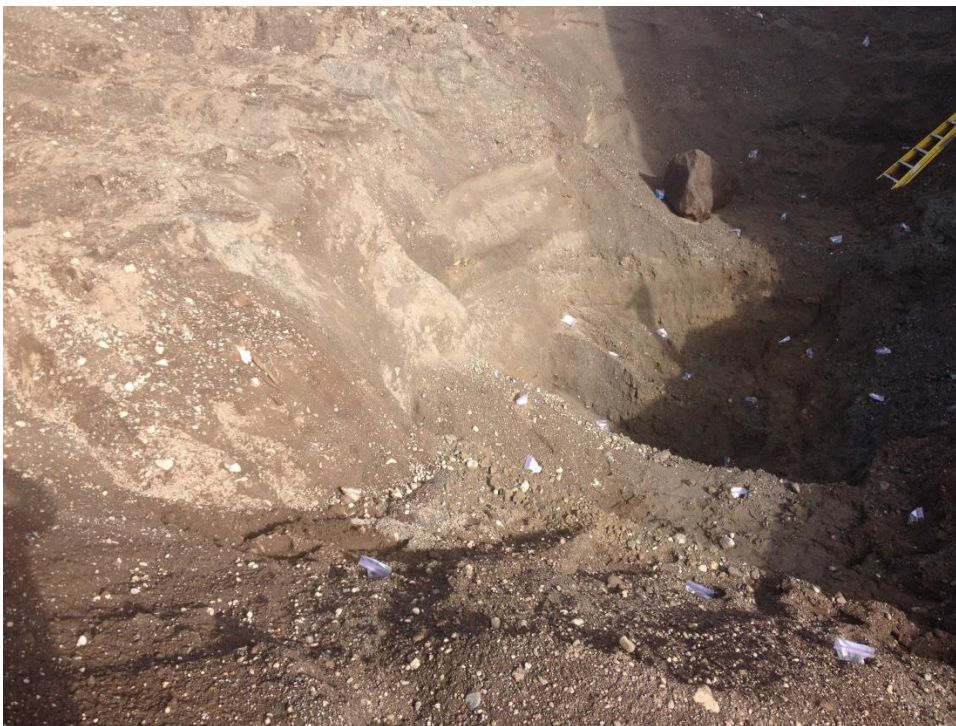
Photo 6 – A large boulder was uncovered during the excavation. The depth of the hole was approximately 17' deep at the deepest tier.
